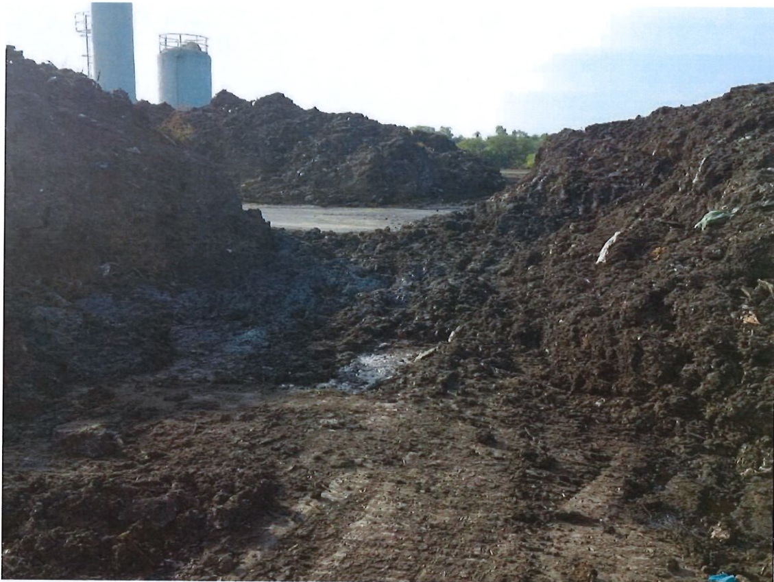
Picture 4. Looking south from the central portion of the southeastern section of the pad. The pad asphalt has been damaged and a hole is located in the central portion of this picture. The rock below the asphalt is exposed.
