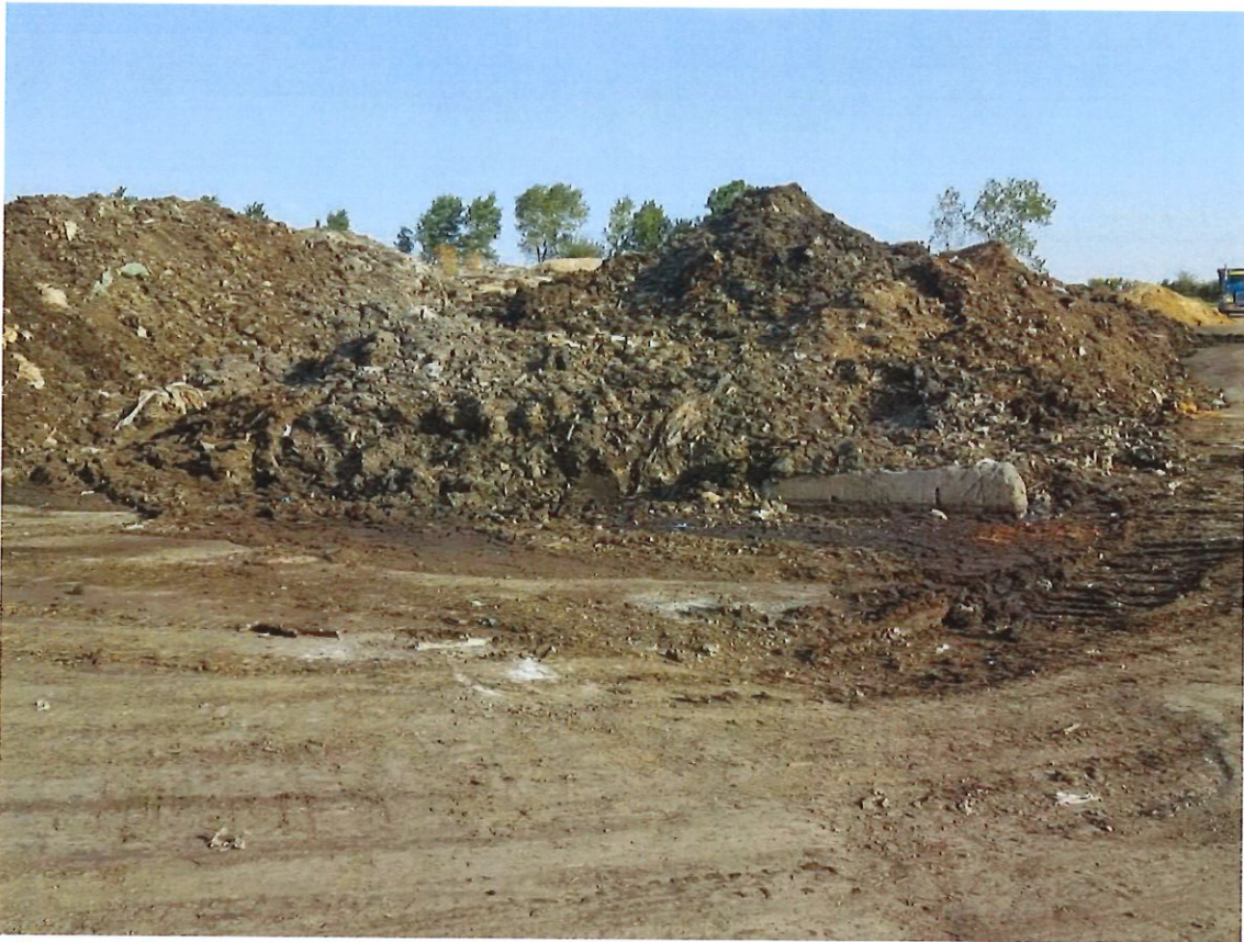
Picture 3. Looking north from the east-central portion of the pad. The drain next to the concrete block, on the middle-right of the picture, remains blocked.
