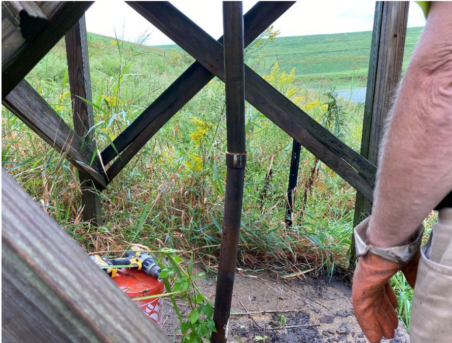
Photo 9: PVC of MW-17 was bent. (Looking north)
