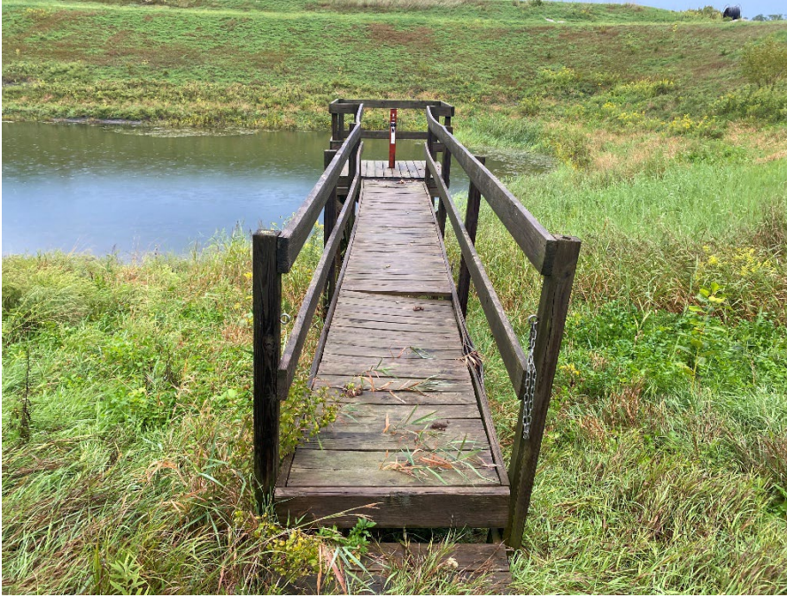
Photo 3: Condition of boardwalk to well prior to well abandonment. (Looking east)
