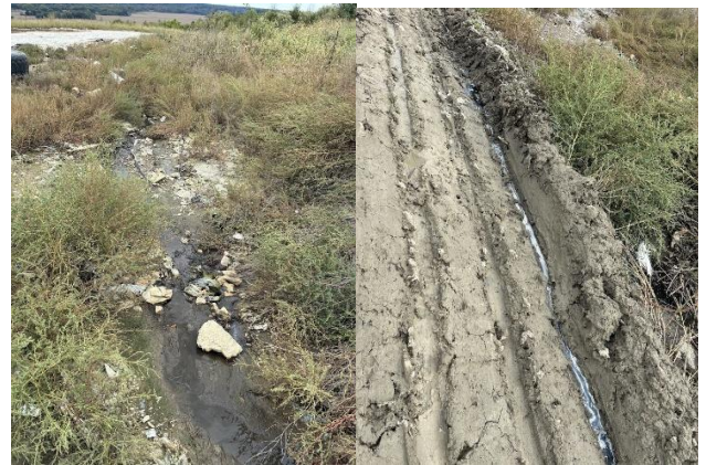
south end of west side - leachate seep
