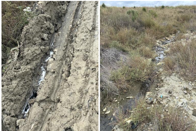
south end of west side – leachate seep
