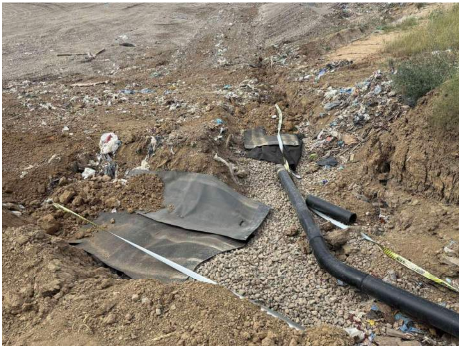
Photo 8: Final noted conditions at the branch off point for HEW – 8 & 9. Grading is completed west of gravel drain windows.
