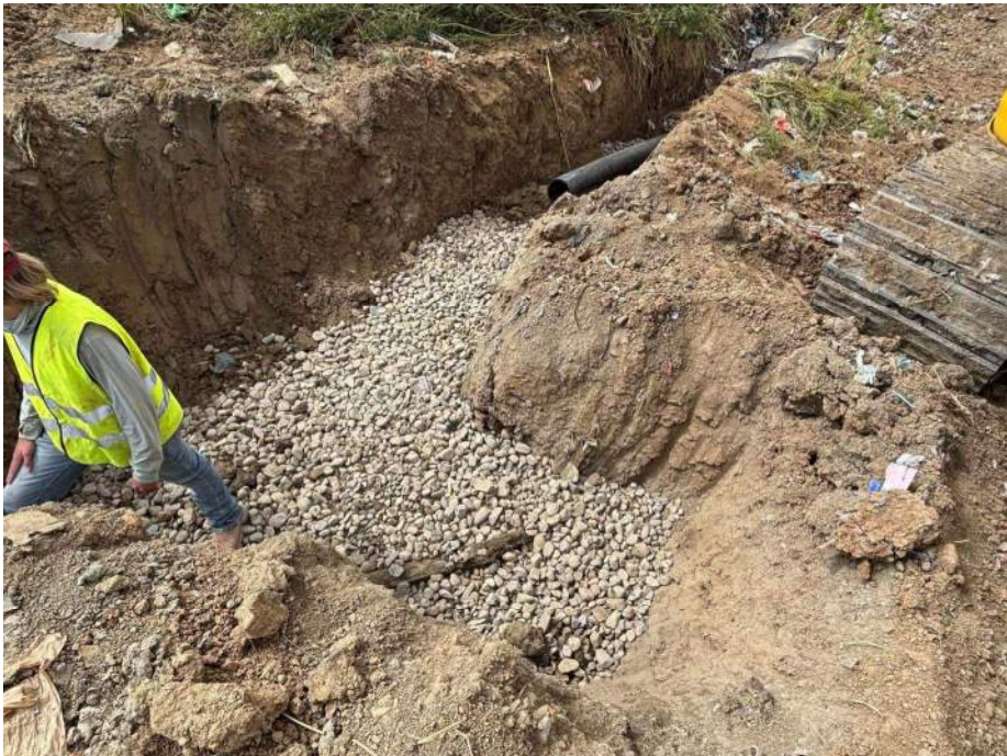
Photo 4: HEW – 10 gravel drain window.
