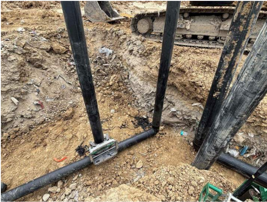
Photo 5: Two 6" risers are attached to GEW-87's riser. Both are positioned adjacent to the 2 solid 8" pipes. Risers are secured with a slip cap. Crew cannot locate enough 8" caps for the 8" pipes and are covered with duct tape.
