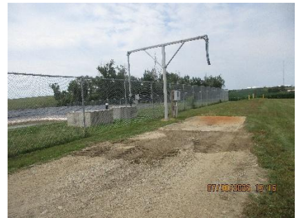
leachate loading rack
