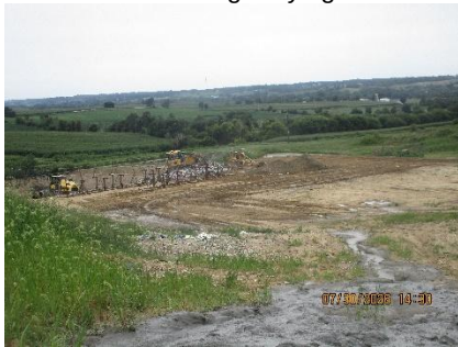
car wash sludge drying area
