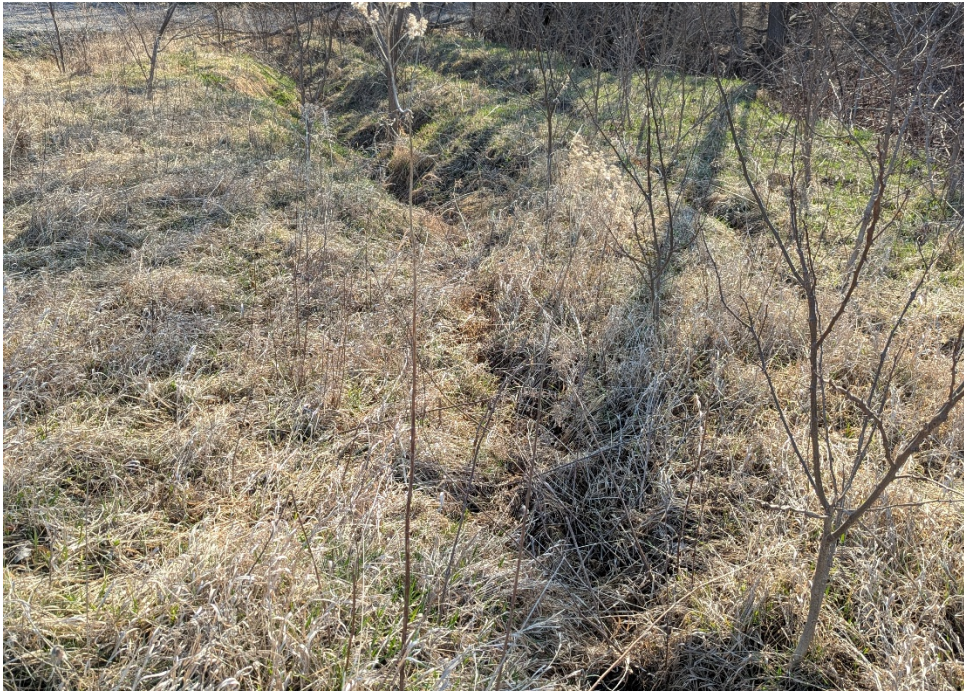
Photo 1: Woody vegetation and erosion rills in the southeast corner of the closure area.
