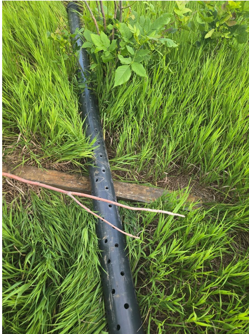
Photo 2: Perforations on gas collection piping.
