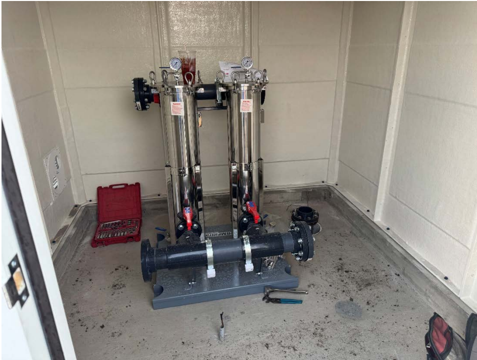
Photo 27: Filter bag skid installed in Treatment Building.
