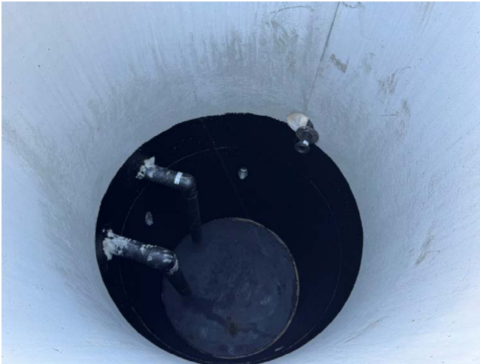
Photo 22: Interior of LS-1 prior to pump installation.
