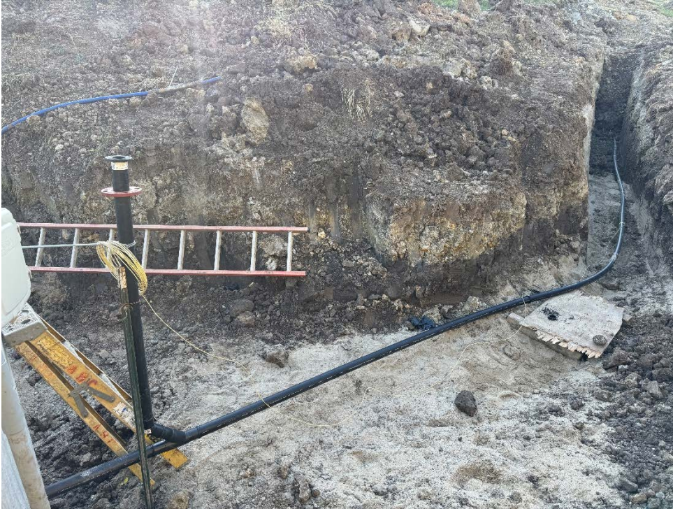
Photo 21: Cleanout and force main installation at discharge from North Lift Station, LS-1.
