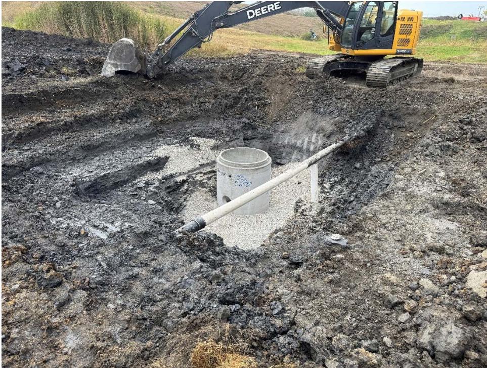
Photo 7: Valve manhole (VMH-1) installation north of Sedimentation Pond. Exposed leachate transfer pipe in foreground.
