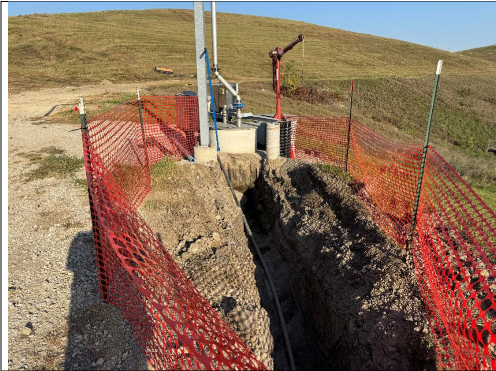
Photo 5: Treatment building floor drain piping to GU-EX.
