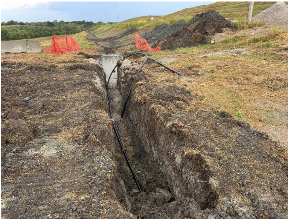
Photo 8: Air/vacuum release valve manhole and force main installation in trench with tracer wire.
