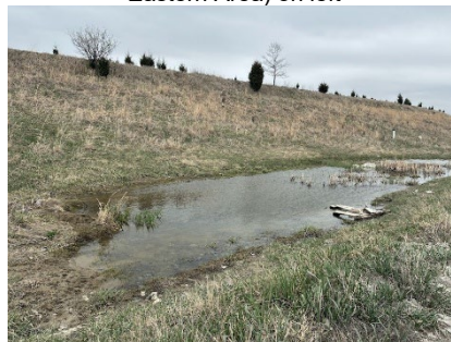
Ponding near western leachate lagoon access road on east side of roadway
