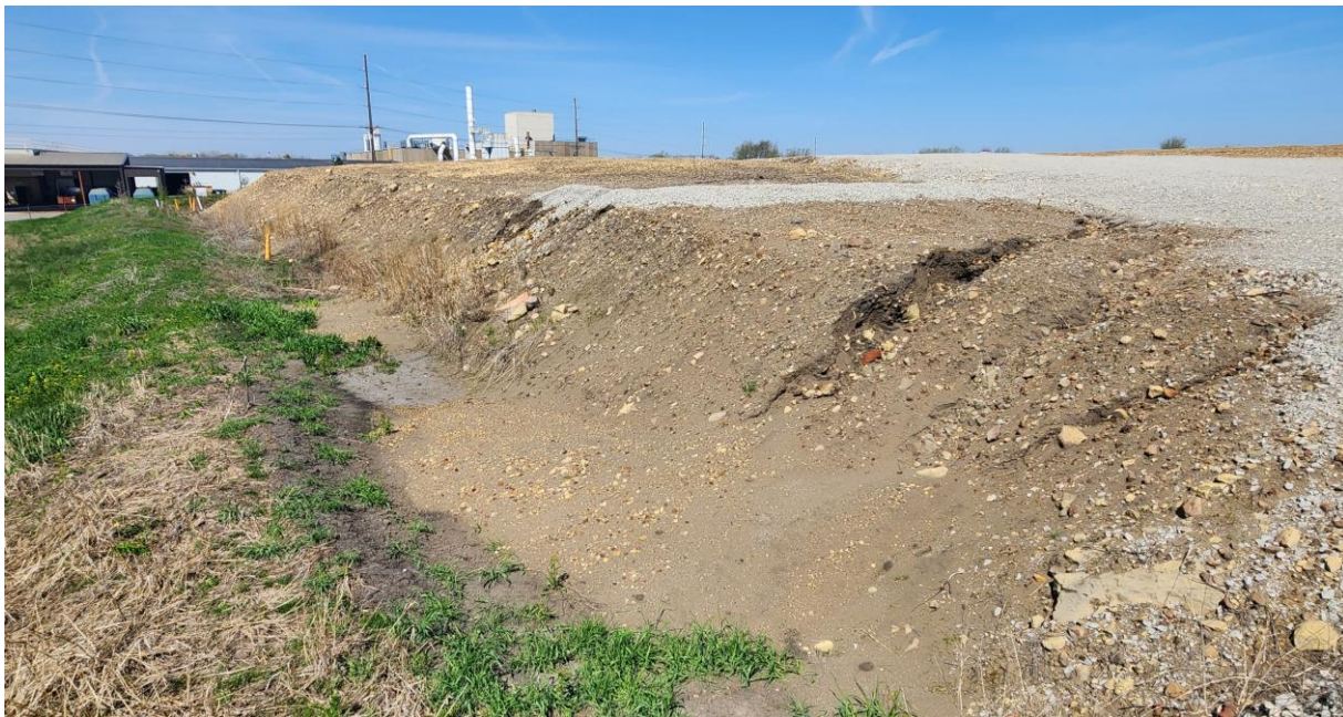
Photo 2 Area of foundry sand erosion into the low-lying perimeter of the cell. No evidence of a release outside the cell was observed.
