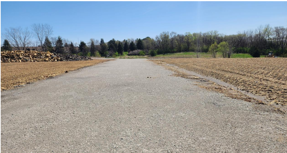
Photo 6 Gravel access road with crushed foundry sand near elevation of road surface. Staged blocks before brushing in the background. Looking east.
