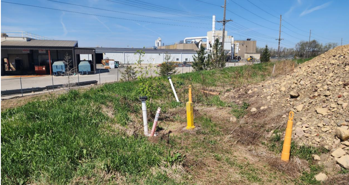
Photo 3 The far white leachate clean-out riser was repaired since the October 2025 inspection. Photograph also shows one of the two woody saplings slated for removal.
