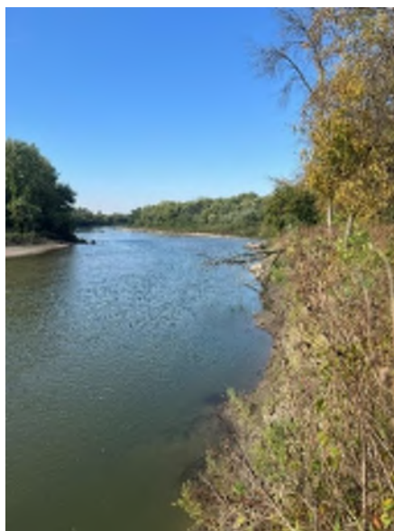
Figure 8: Looking upstream to the west at the concrete slabs on the left bank
