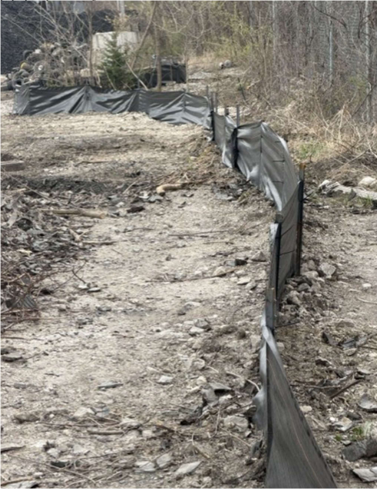
New Silt Fence Installation West property at top of hill facing South
