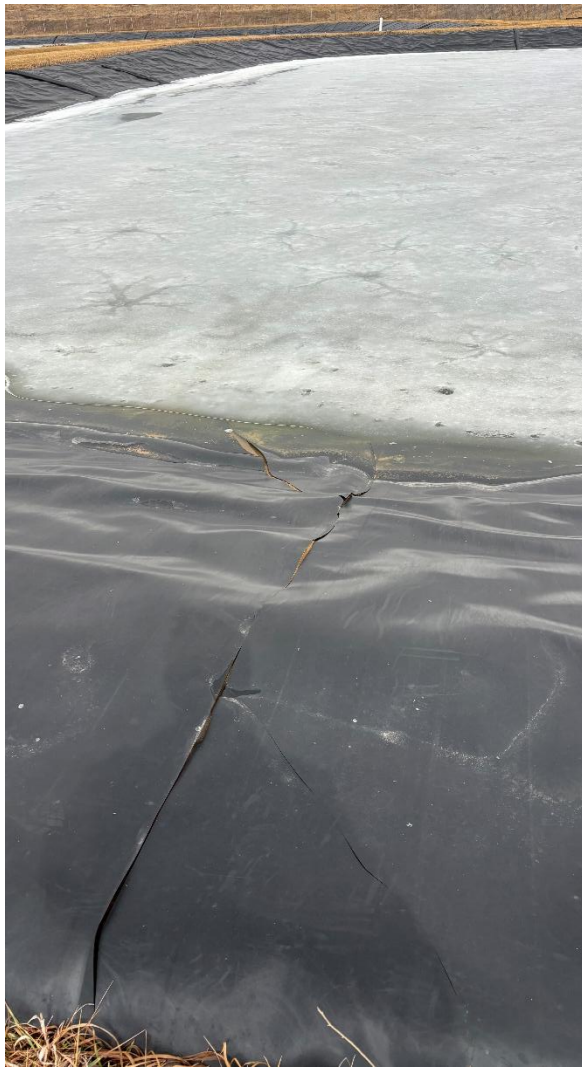
Photo 1: Damage in 1991 lagoon, looking north, 03-09-26.
