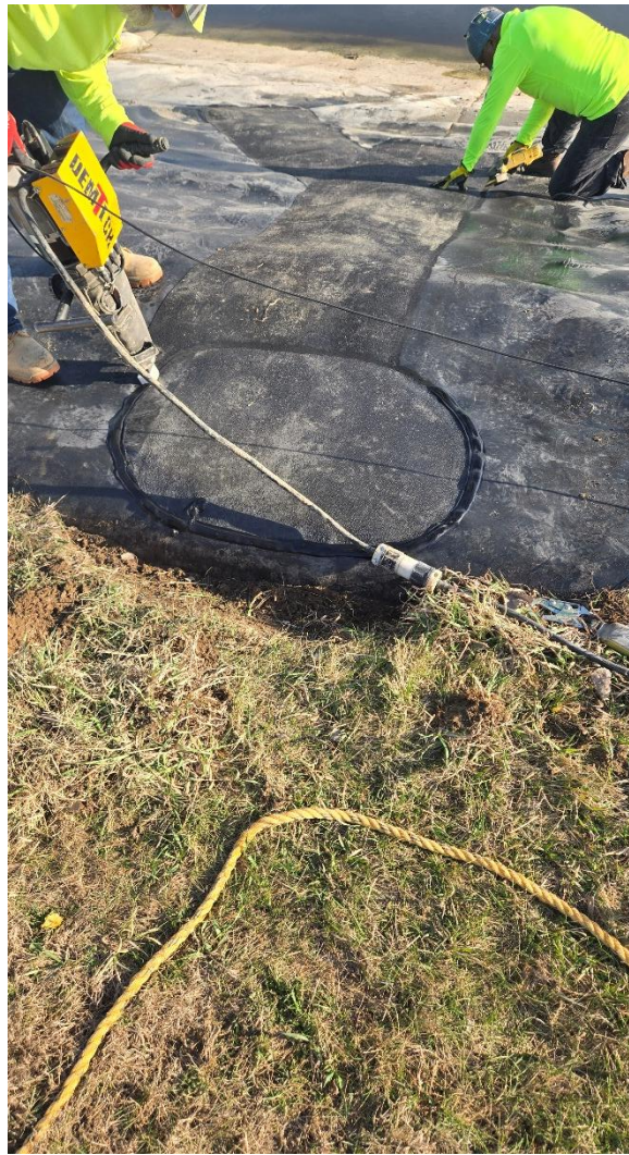
Photo 3: Grinding and extrusion welding patch in 1991 lagoon, looking north, 03-30-26.
