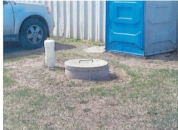
Load Out Pit Pump Out
