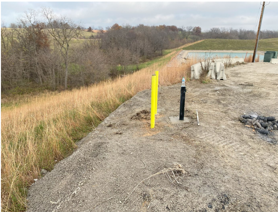
Photo 4: Completed MW-125. Photo facing North. Concrete barriers were replaced by site staff following completion of well installation.
