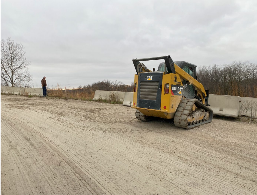
Photo 1: Moving concrete barrier to access drilling location for MW-125. Photo facing Southwest.
