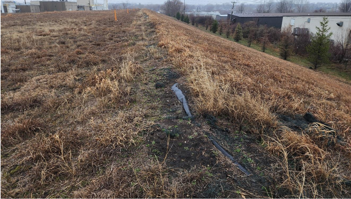
Photo 9 4/1/2024. North area of landfill, facing west, showing exposed membrane (not part of the cover).
