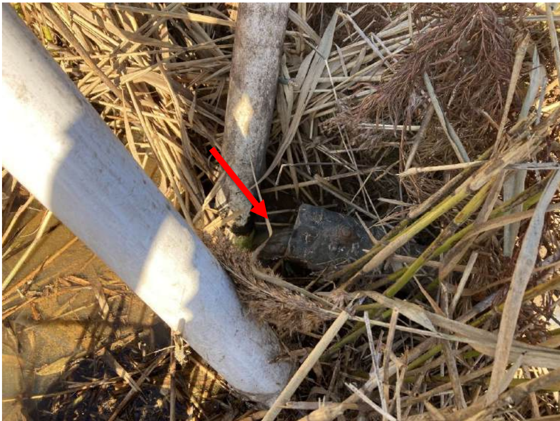
Free flowing water at outlet (during lateral jetting)
