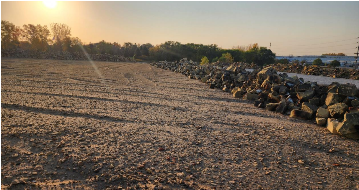
Photo 6. Looking southeast over previously crushed foundry sand with staged molds placed along the gravel access road shown to the right.
