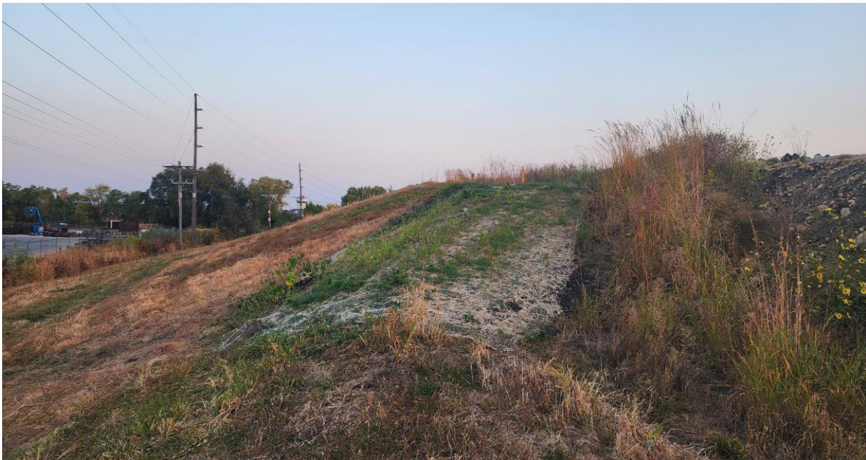
Photo 2. West side of landfill (looking north) at edge of closed section showing recently reseeded and matted area.
