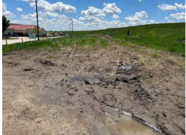
Drainage and grading issue near the leachate tank, facing south.
