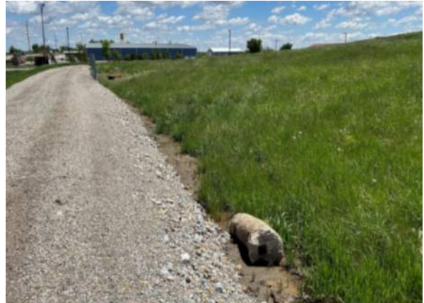
Drainage/grading in the interior ditch of the final cover access road, facing southeast.
