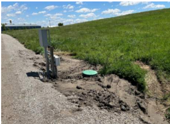
Drainage problems near leachate well, facing southeast.
