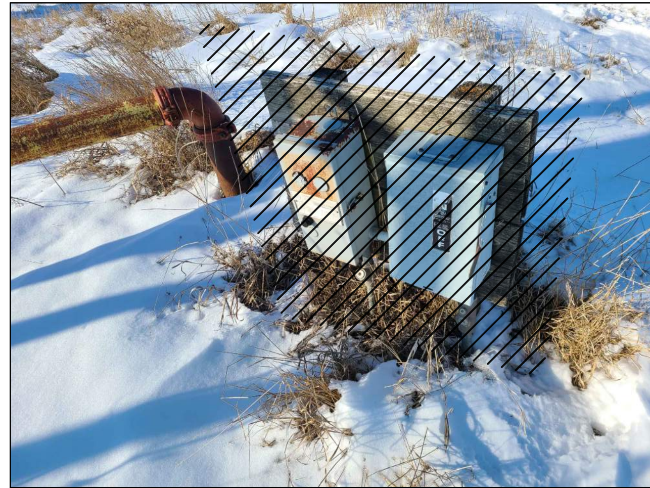
3 EXISTING LEACHATE LOADOUT DISCONNECT AND STARTER
