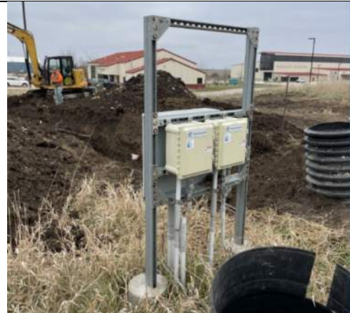
Electrical panel near leachate storage tank, facing east.
