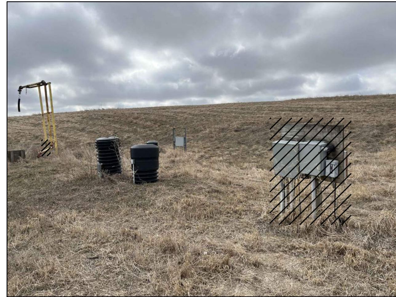
2 EXISTING EQUIPMENT RACK AND LEACHATE LOADOUT PUSHBUTTON
