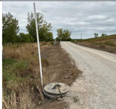
Final cover access road encroaching on leachate well, facing north.
