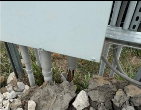
Broken electrical on LW-8, facing south.
