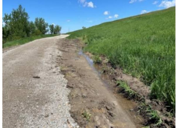
Drainage issues in the interior ditch of the final cover access road, facing north.
