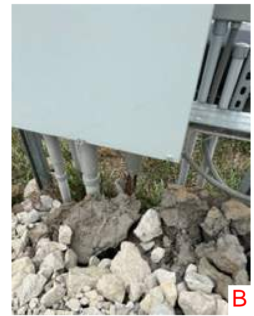
1A - Fill around electrical panel and grade area to drain 1B - Repair broken electrical conduit
