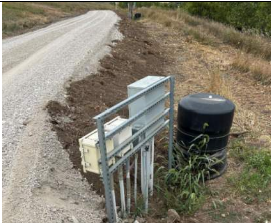
Additional fill placed on the west side of final cover access road, facing south.
