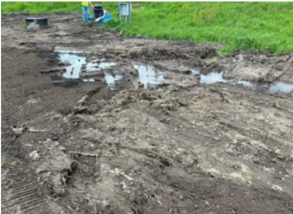
Ponded water near the leachate storage tank, facing southwest.
