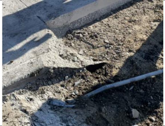
Chipped corner of existing concrete, facing southeast.
