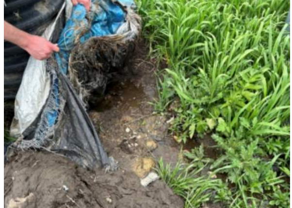
Leak near the new check valve, facing south.
