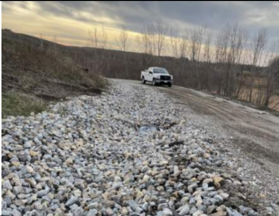
Riprap installed on interior ditch of final cover access road without v-ditch, facing southwest.
