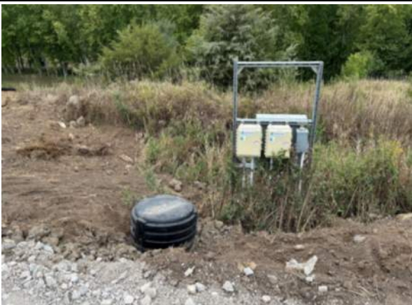
Final cover access road grading drainage not adequate around leachate well, facing west.
