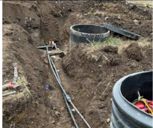
Installed leachate bypass system, facing northeast.
