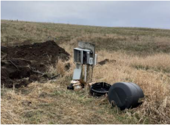
Abandoned electrical panel near the leachate storage tank, facing west.
