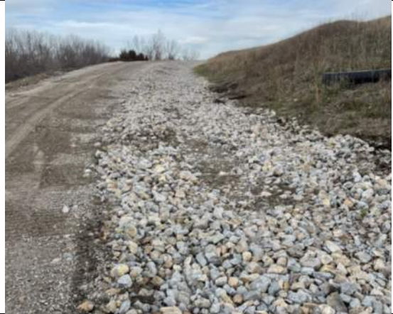
Riprap installed on interior ditch of final cover access road without v-ditch, facing northwest.
