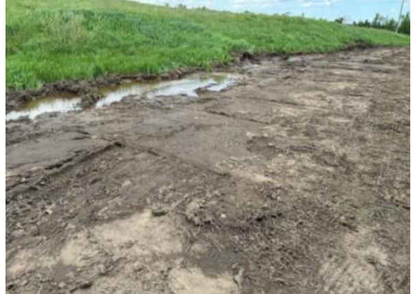
Ponded water near the leachate storage tank, facing northwest.
