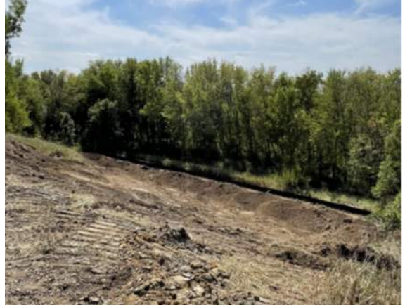
Grading on the slope west of the final cover access road, facing southwest.
