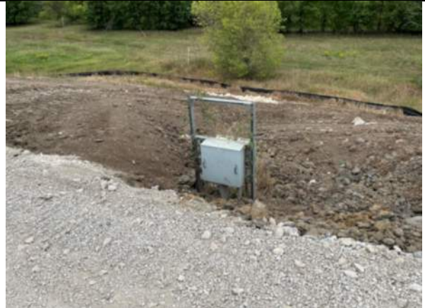
Final cover access road grading drainage not adequate around leachate well, facing west.
