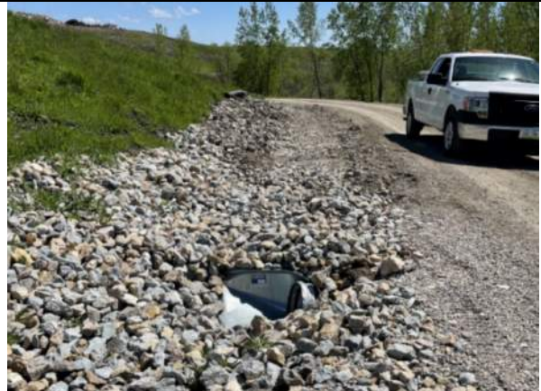
V-ditch missing in interior ditch, facing south.
