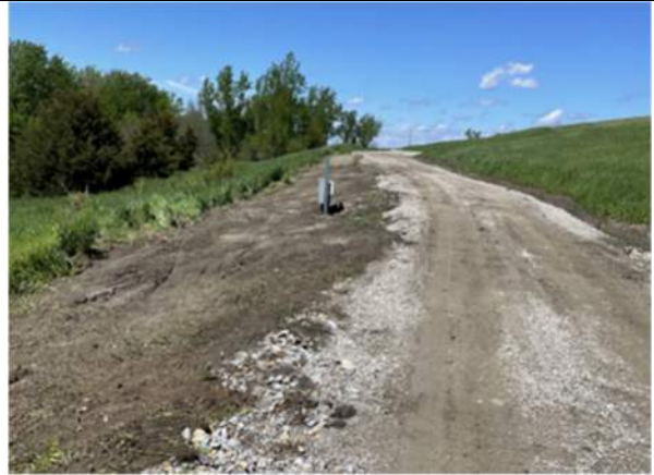
Slope of final cover access road on the southwest portion of the roadway, facing northwest.
