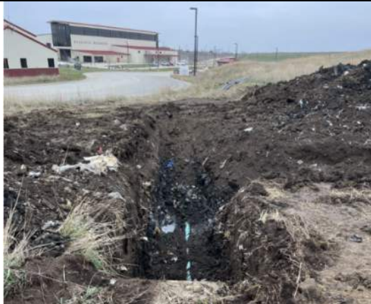
Existing leachate forcemain exposed south of the leachate storage tank, facing southeast.
