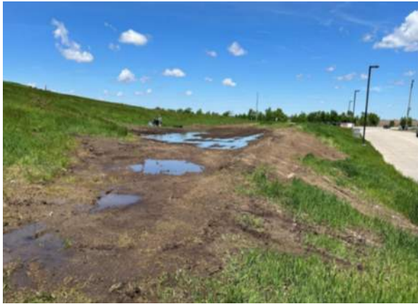
Drainage and grading issue near the leachate tank, facing north.
