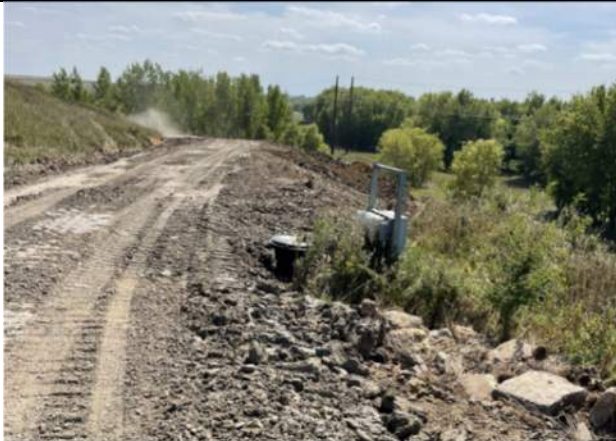
Final cover access road crowding leachate well, facing south.
