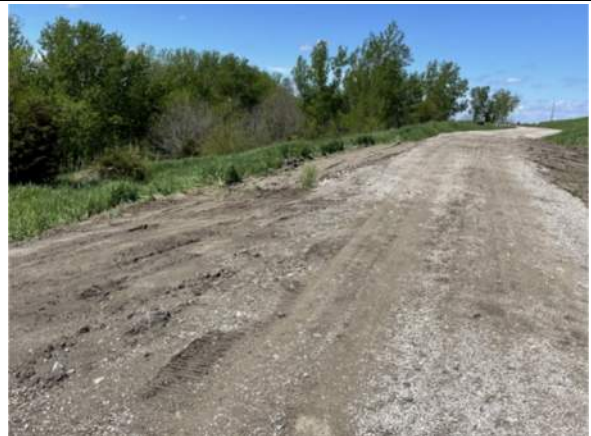
Slope of final cover access road on the southwest portion of the roadway, facing northwest.
