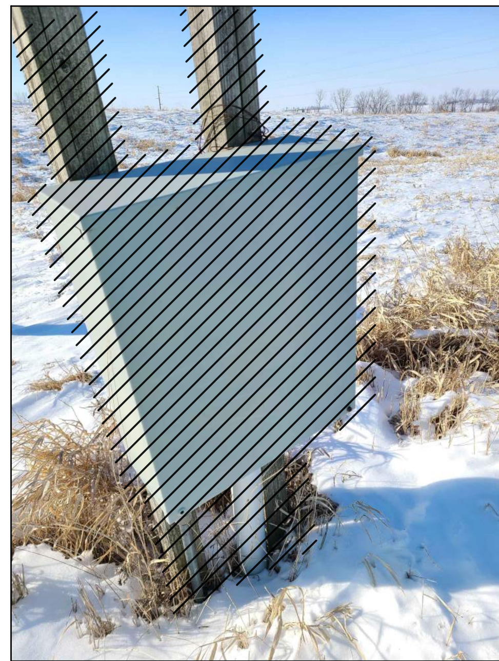
1 EXISTING UNDERGROUND STORAGE TANK ELECTRICAL EQUIPMENT
