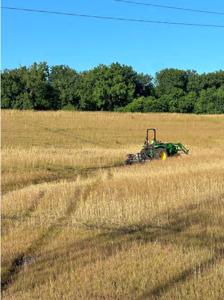
Photo 4: Fine grading rutting areas on Main Ash Pond Closure Area (looking southwest).
