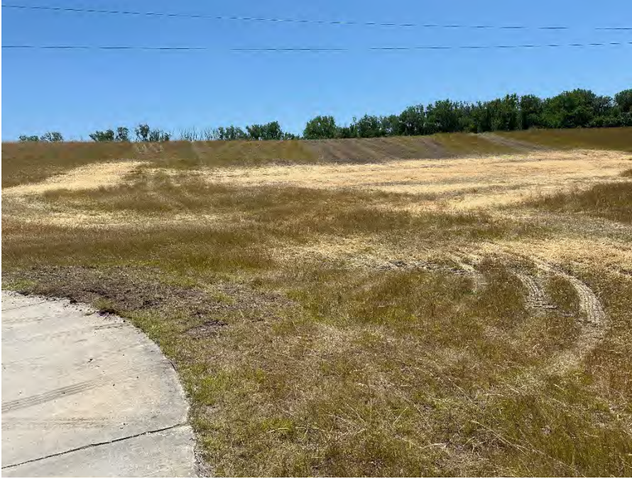
Photo 6: Precision began placing seed and mulch over areas in the Main Ash Pond Closure Area (looking south).
