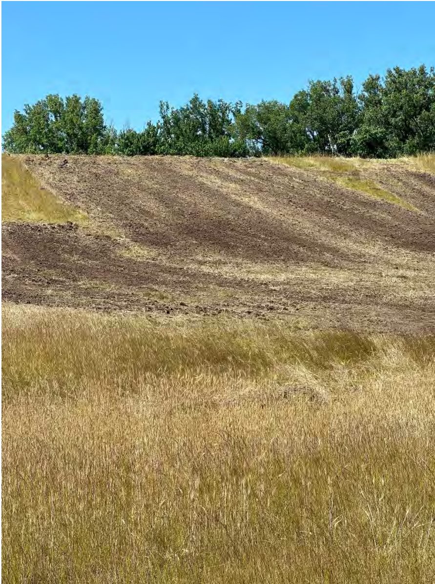
Photo 5: Topsoil placed from ramp area over damaged area in Main Ash Pond Closure Area to reach 6-inch thickness (looking south).
