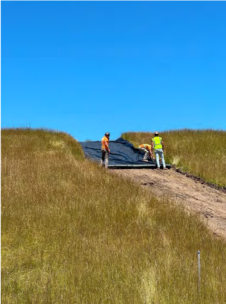
Photo 2: Placing surface course aggregate on geotextile for ramp (looking northwest). Installing geotextile on top of low-permeability clay cover material for ramp (looking southeast).
