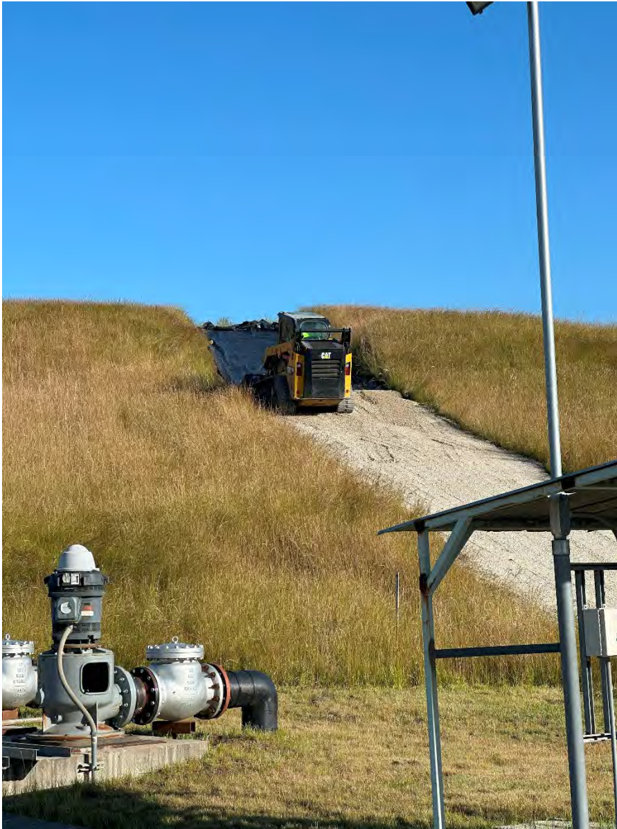
Photo 3: Placing 6 inches of surface course aggregate on geotextile for ramp (looking northwest).
