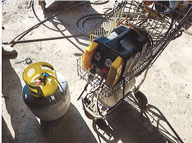
Photo 3: Refrigerant and removal machine
