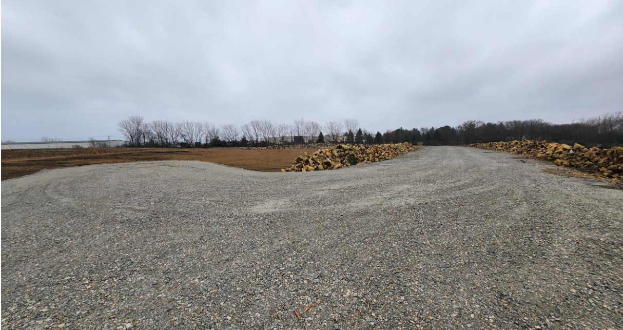
Photo 1. View of new access road from the west edge of the road, looking toward the entrance (southeast). Staged blocks placed on either side of the access road.
