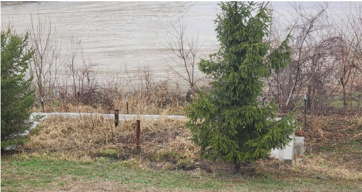
Photo 2. Area of new retaining wall around MW-8 and MW-13 on north side of landfill. Overgrown brush observed in October 2023 is now cleared.
