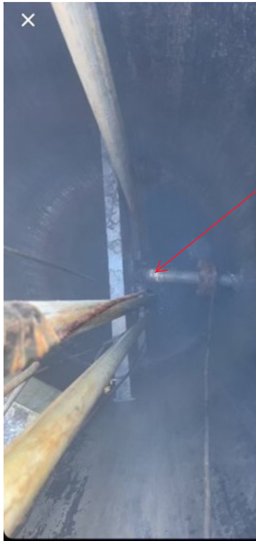
FIGURE 3 A1 UNDERDRAIN DISCHARGE AT CELL A GROUNDWATER EXTRACTION MANHOLE
