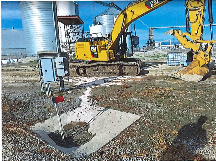
Photo 3: Spilled area looking north from valve area
