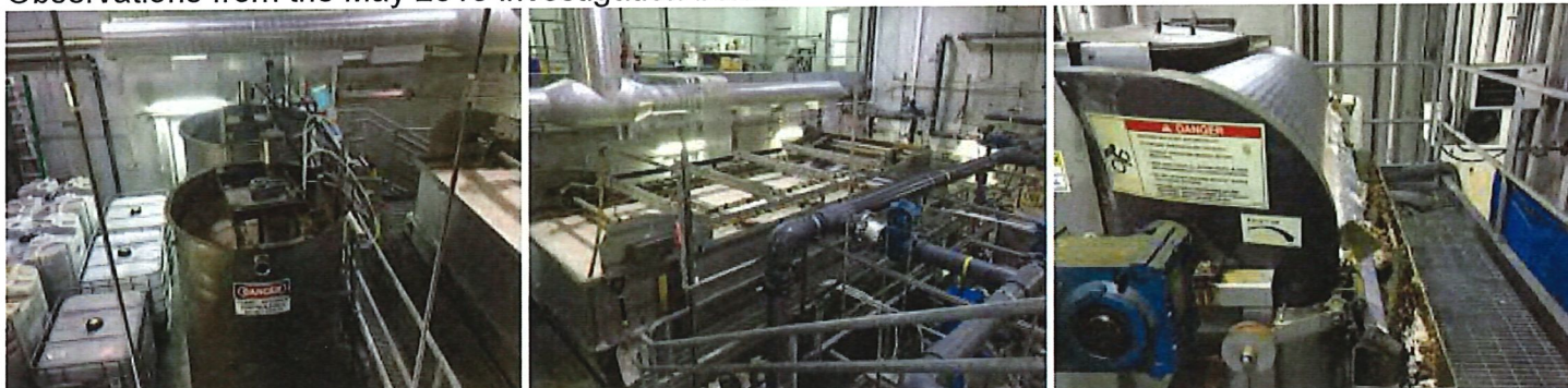
Photos 5 -7: Looking at the equipment associated with the DAF
