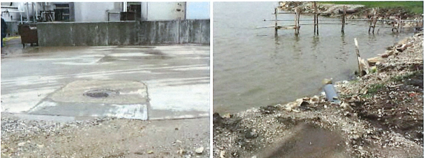
Photos 1 and 2: Looking at the sealed manhole and the emergency outlet to the north lagoon
