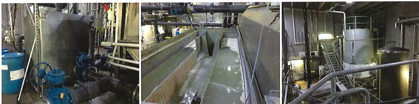
Photos 8 -10: Looking at the equipment associated with the DAF
