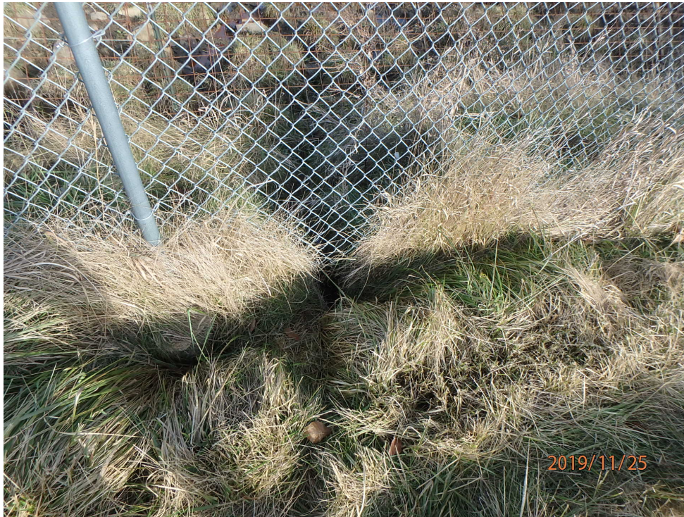
Photo 15 – View of area where water has run under the north fence east of the rip-rap lined drainageway.
