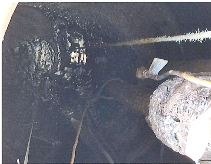
Photo 9: Influent to wet well
