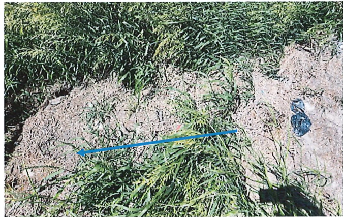
Photo #4: South side of basin with evidence of overflow on berm and dead grass present
