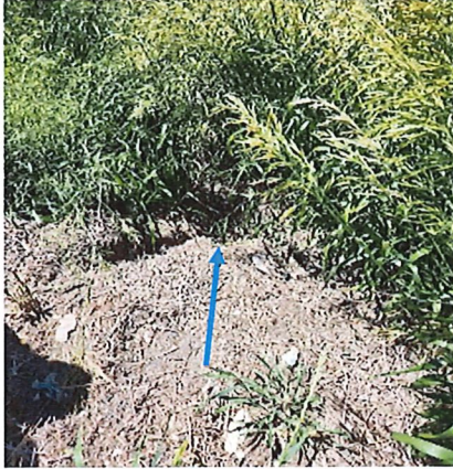
Photo #5: Looking south down the retention basin berm showing erosion and dead grass present
