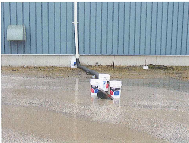
Tile intake plugged with bucket (background). Solid tile now diverting water away from the building and tile intake.
