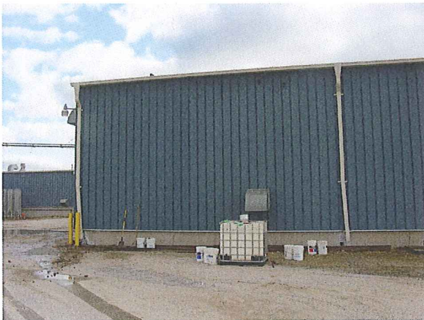
Building where spill occurred Note: tote of recovered product
