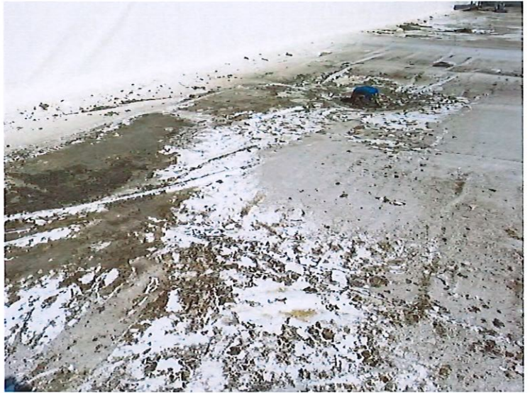
View area of roof near EP-5 showing gelatin debris on the roof.
