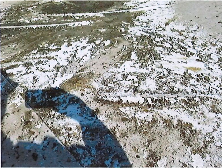
View area of roof near EP-5 showing gelatin debris on the roof
