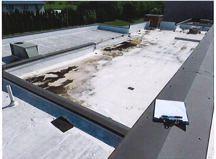
View looking northeast from the roof over the Boiler Rooms at the roof over the office area showing gelatin material on the top of the office roof.
