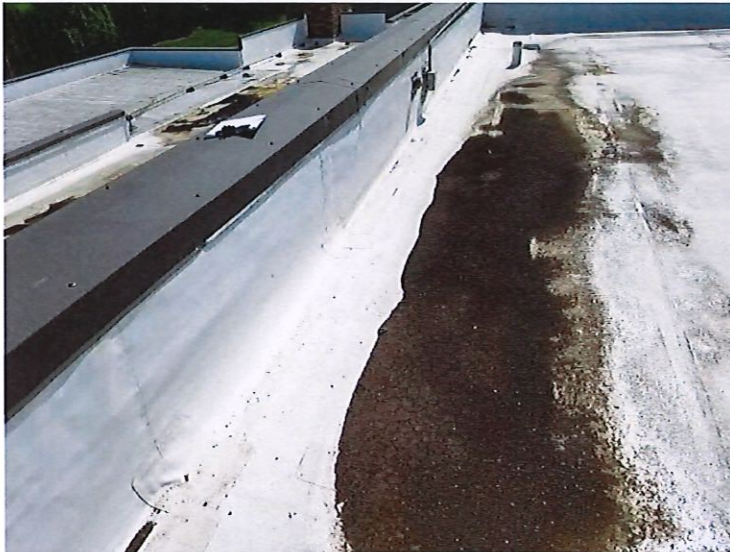
View looking east along the north edge of the roof over the Boiler Room.
