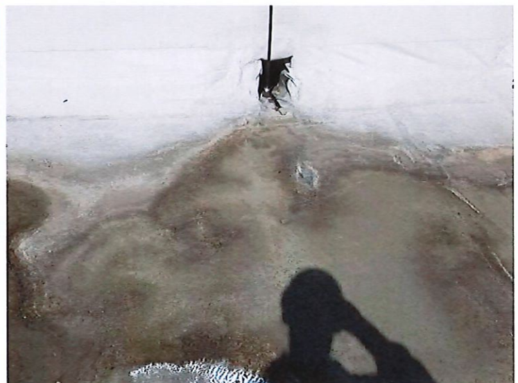
View looking west at roof drain inlet in the northwest corner of the roof near EP-12.
