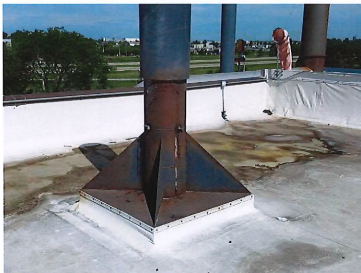
View looking northwest at area of roof around EP-12 showing gelatin material along the west edge of the roof.
