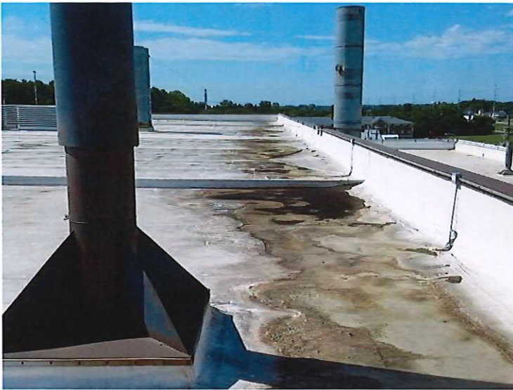
View looking south from EP-12 (left stack) along the west edge of the roofline by EP-12. EP-18 and EP-19 can be seen in the background (from left to right, respectively).
