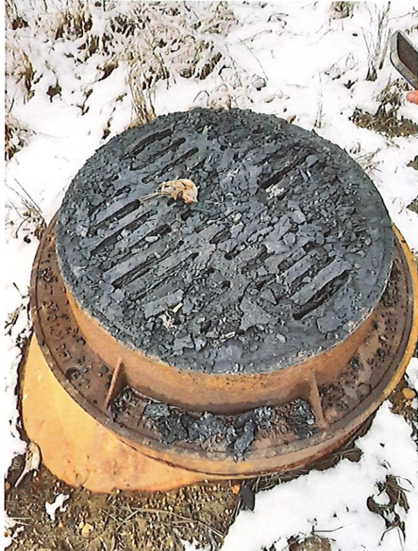
Picture 3. Corrosion and dead bird on manhole cover
