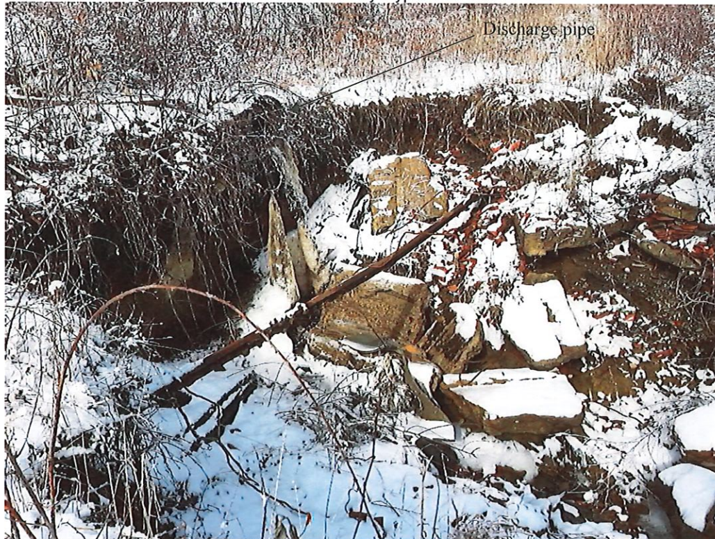
Picture 4. Discharge from Sediment Basin to Gully/Gypsum Creek
