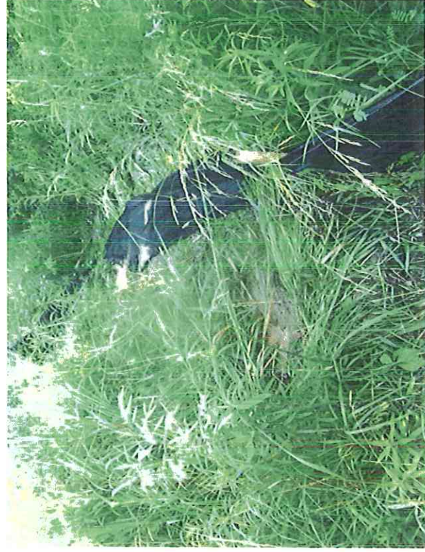
Picture 4: Additional photo of silt fence on NE corner. The silt fence was not properly installed (not trenched in).
