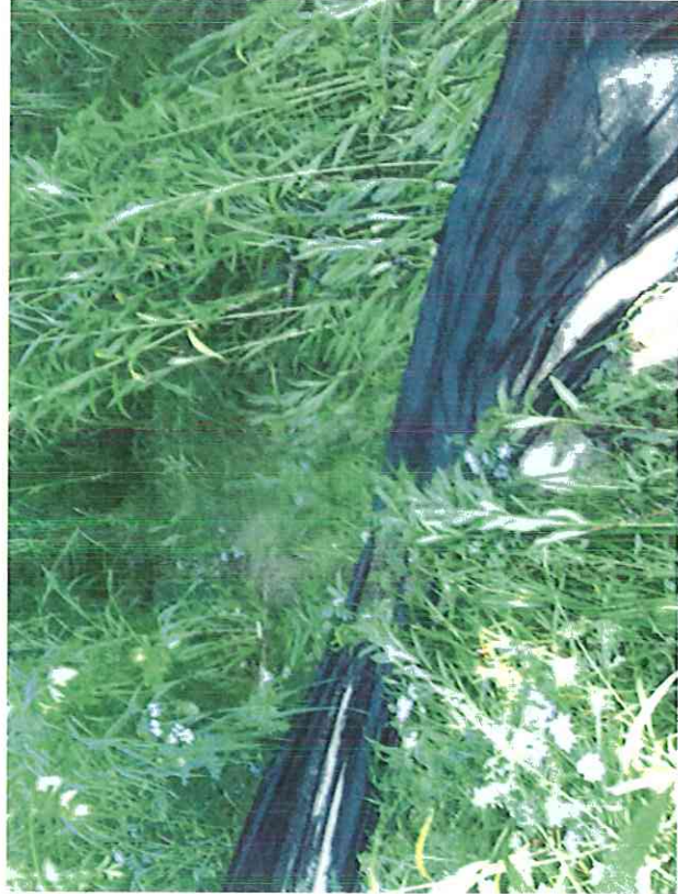
Picture 3: Silt fence downslope of the gully on the NE corner. Sediment has topped fence and continued to migrate north.
