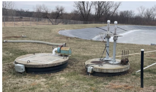
valving and lift station
