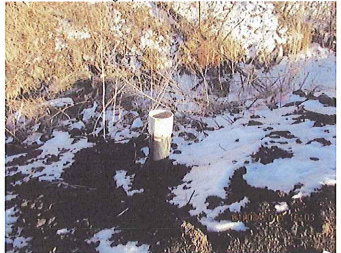
gas venting at east toe of north filled area
