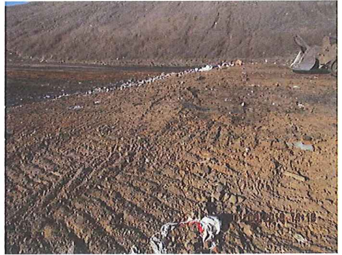
working area in Cell 2
