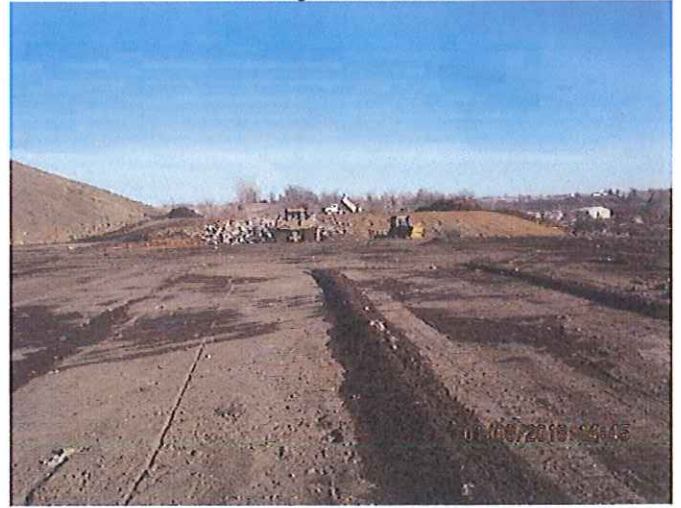
working area in Cell 2
