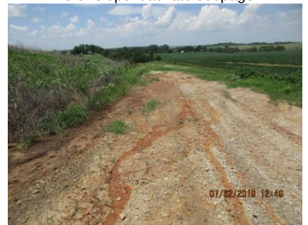
north slope leachate seepage
