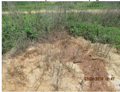
north slope leachate seepage
