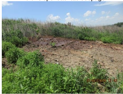
north slope leachate seepage
