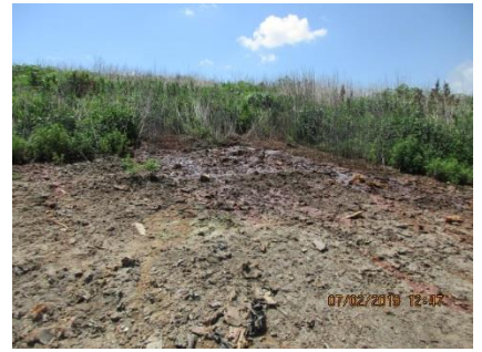
north slope leachate seepage
