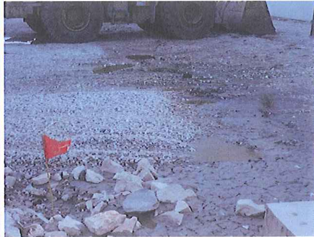
Storm water drain covered with manure.
