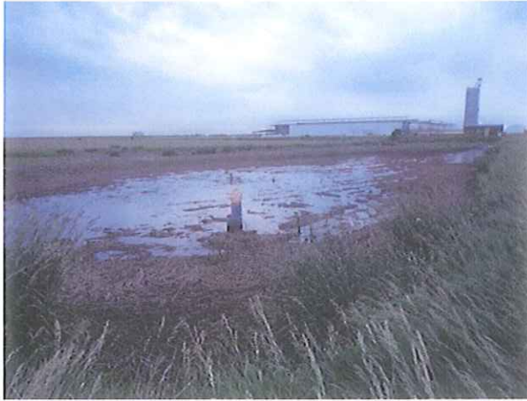
Storm water basin and outlet tube
