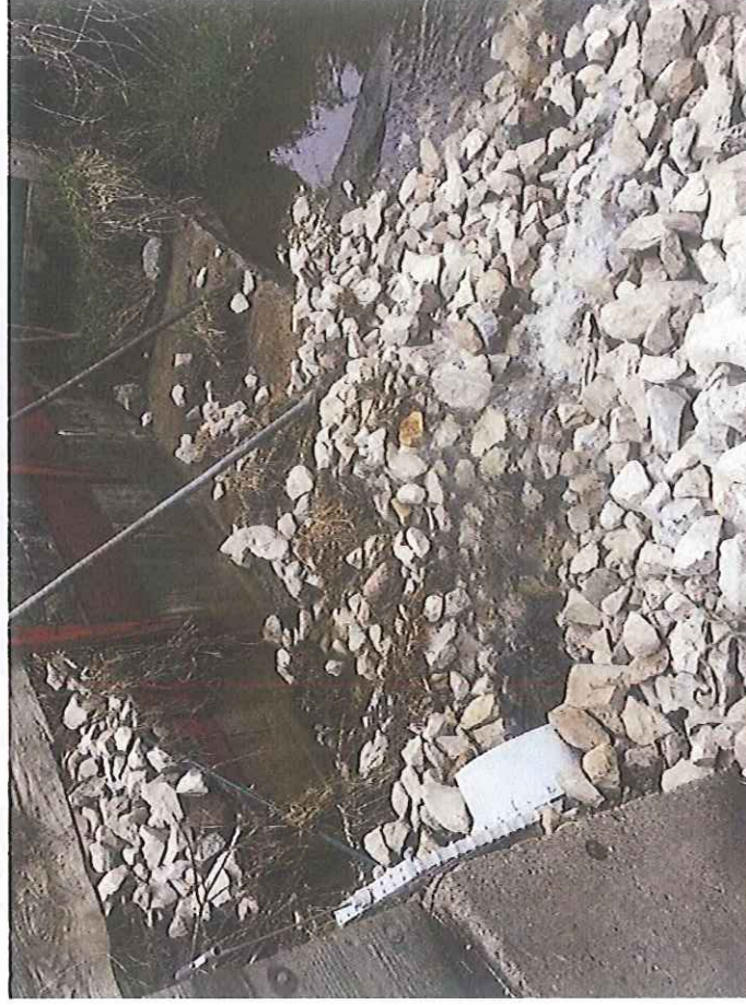
Outfall of waterway at Daybreak Foods showing both tile flow and overland flow. Overland flow over the concrete weir is difficult to observe in this picture due to the limited flow. The tile water is clear. The discolored overland flow is seen on the right side of picture. (05/02/2018)
