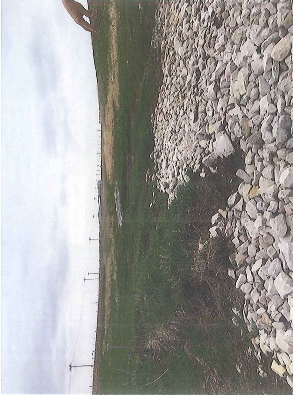
Wastewater ponded in Daybreak Foods waterway visible in center of picture. Wastewater also visible on far right of picture moving through the rocks. Picture taken looking south. (05/02/2018)
