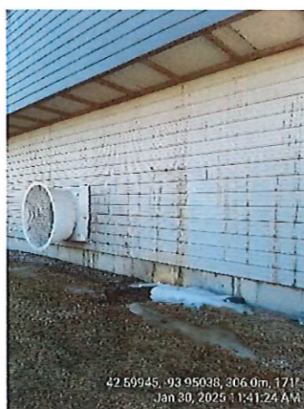
Waterline flush pipe through the wall on the north building.
