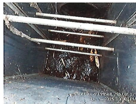
Branches and cornstalks in the control structure.
