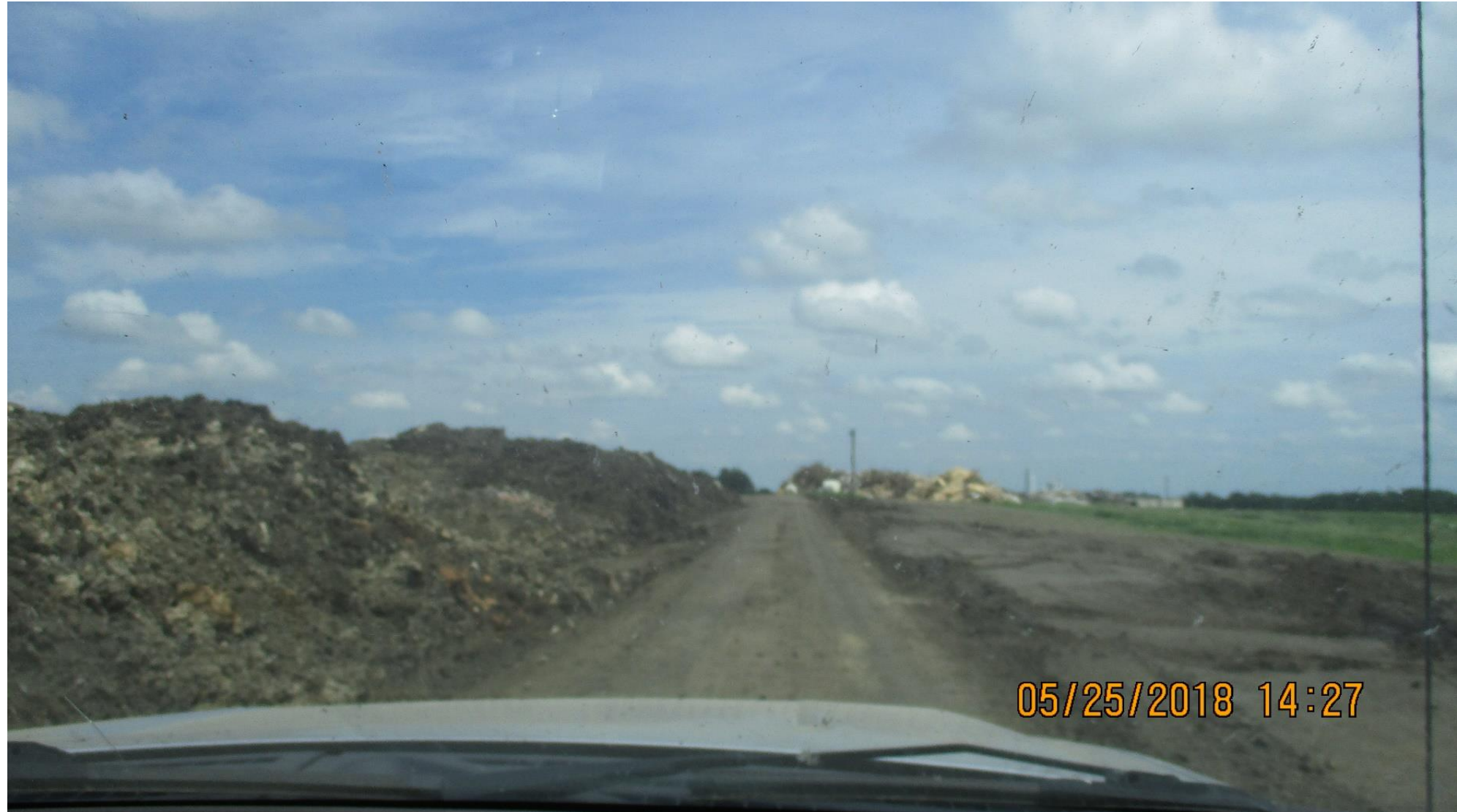
Chamness Technology, Inc. - View of southwestern portion of composting pad looking east
