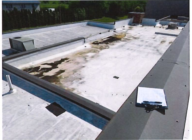
View looking northeast from the roof over the Boiler Rooms at the roof over the office area showing gelatin material on the top of the office roof.
