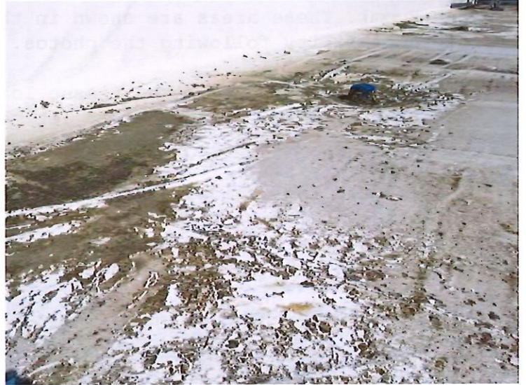
View area of roof near EP-5 showing gelatin debris on the roof.
