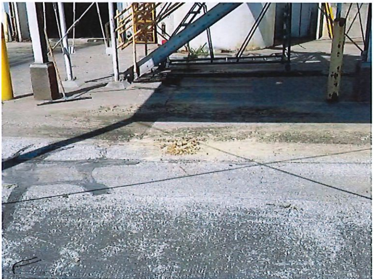
View of small pile of tissue debris located directly below the chute at the tissue loadout (EP-23).
