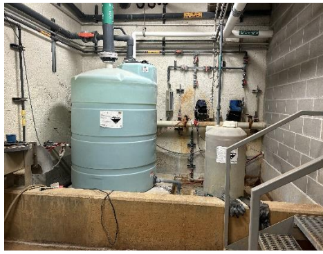
Fluorosilicic acid bulk and day tanks. Piping and chemical feed lines are clearly labeled.
