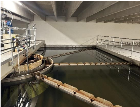
Clarifier on the newer side of the plant.
