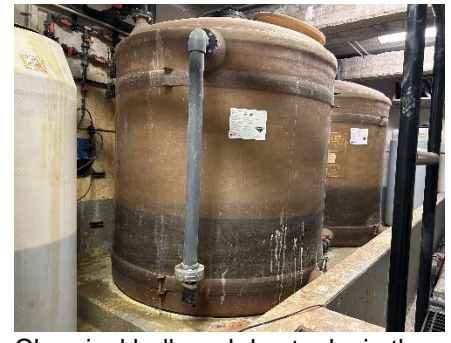
Chemical bulk and day tanks in the basement. The bulk tanks are too large to remove from the basement and are filled via chemical offloading previously pictured.
