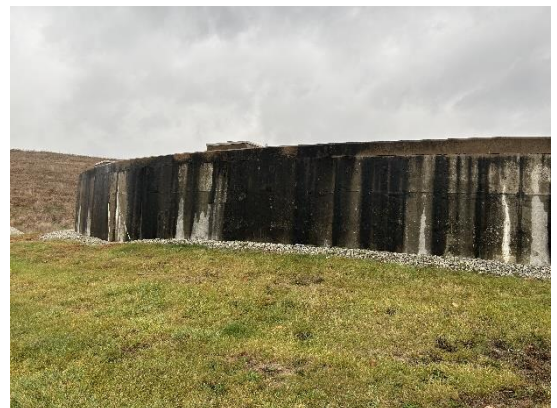
GSR just west of the water treatment plant.
