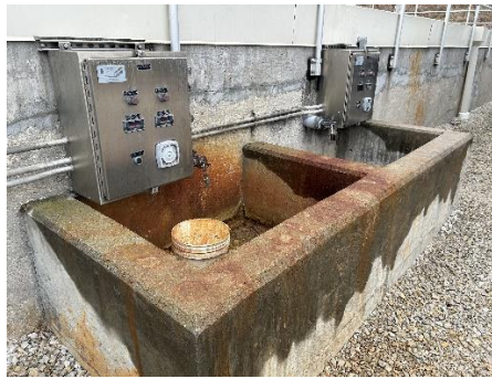
Chemical offloading area with secondary containment and labels outside of the water treatment plant.
