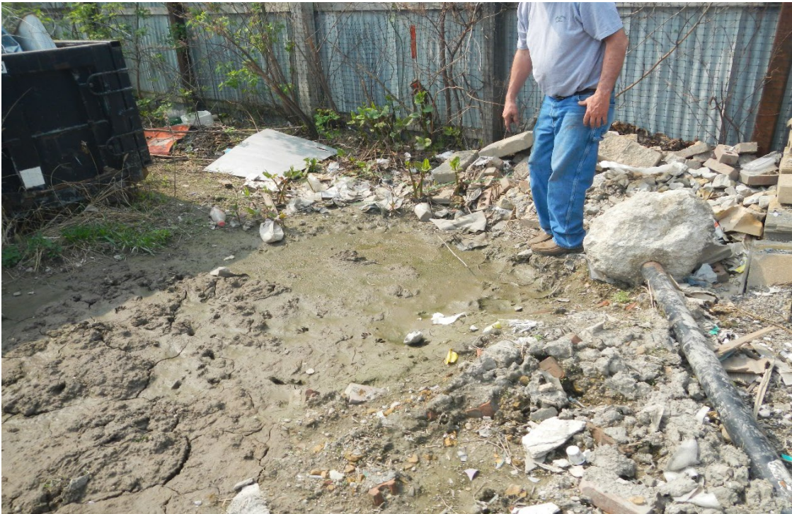
Photo #: DSCN1220, one of the three inlets completely covered with sediment
