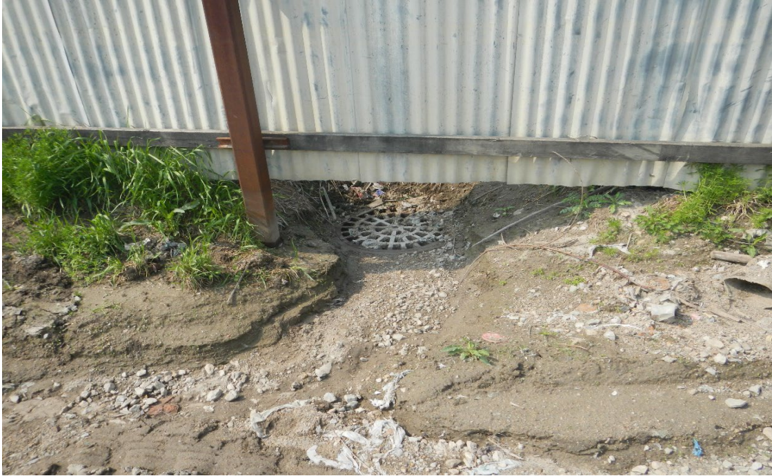
Photo #: DSCN1217, stormwater runoff entering one of the inlet to the MS4
