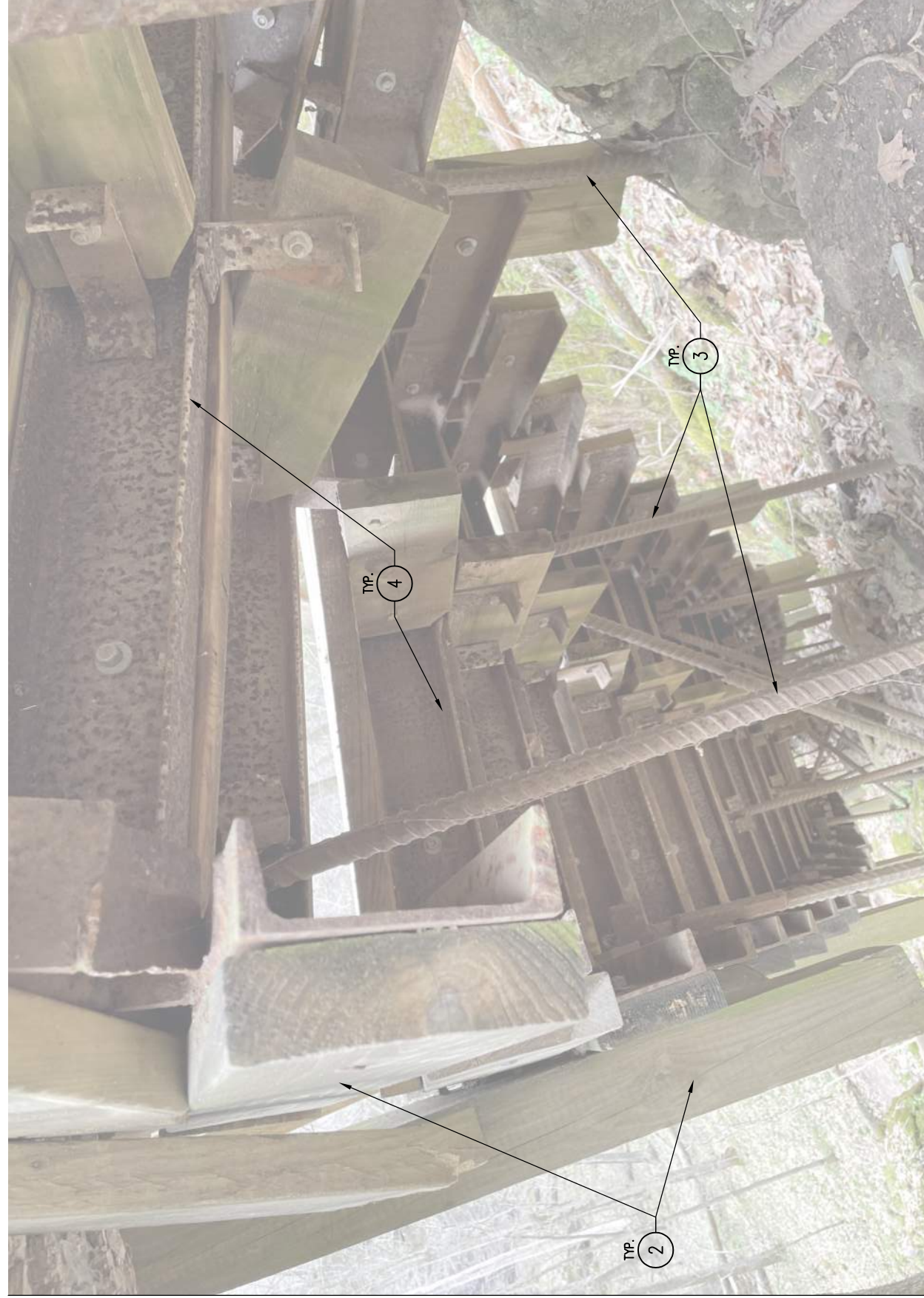
01 BALANCED ROCK PHOTO – UNDERSTAIR DAMAGE
