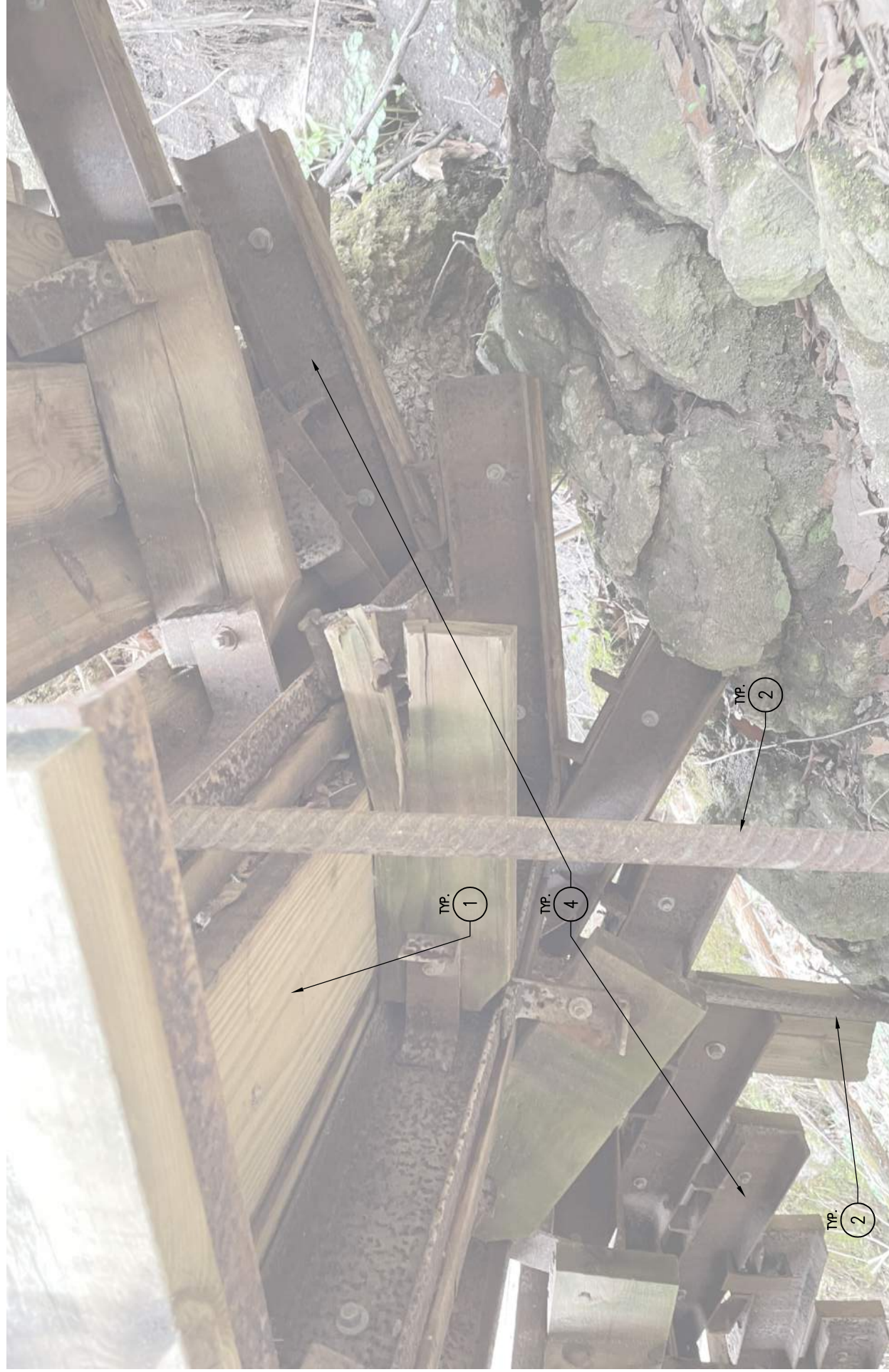
02 BALANCED ROCK PHOTO – UNDERSTAIR DAMAGE
