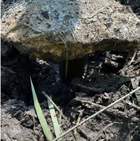
Photo 17: Close up view of excavation under concrete pad during abandonment of WFE-7B.
