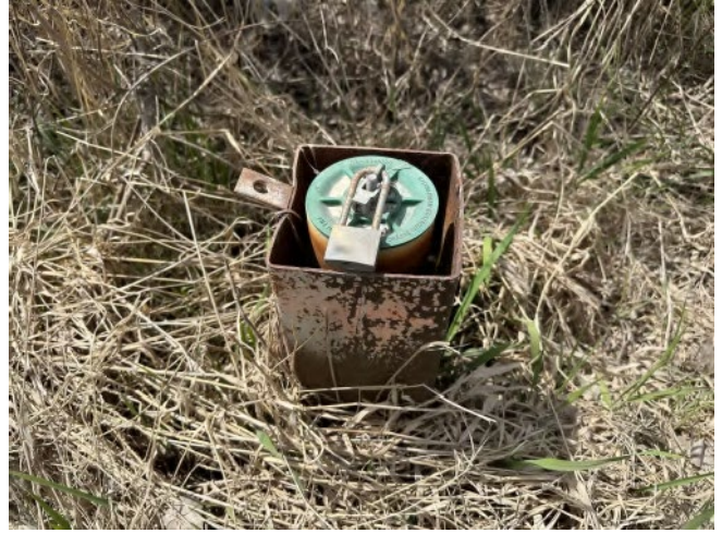
Photo 6: Close up view of WFE-5A with stickup lid missing.
