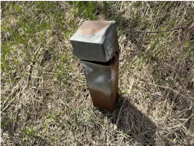
Photo 9: Close up view of WFE-6B showing lid damage facing West.
