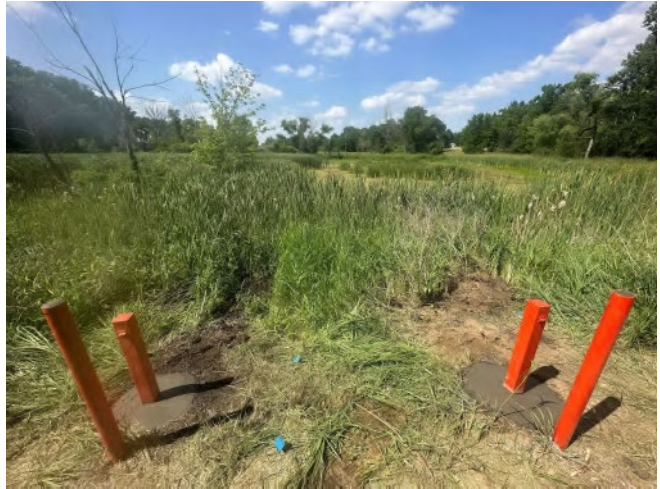
Photo 2: View of WFE-7AR & WFE-7BR post-installation.
