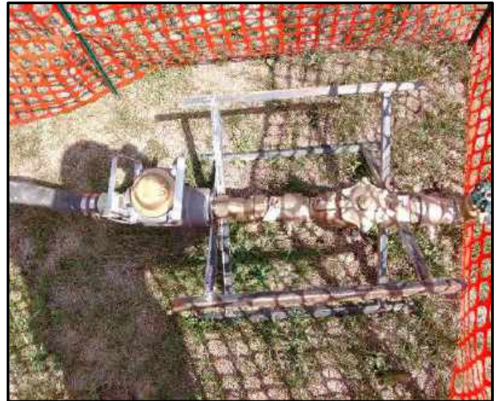
Photo 6: The fire hydrant water meter set up on the corner of 33 rd St and Eastern ave.
