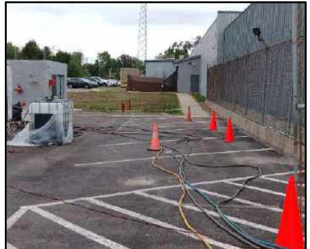
Photo 10: Active injections line running to the On-Site Source Grid.
