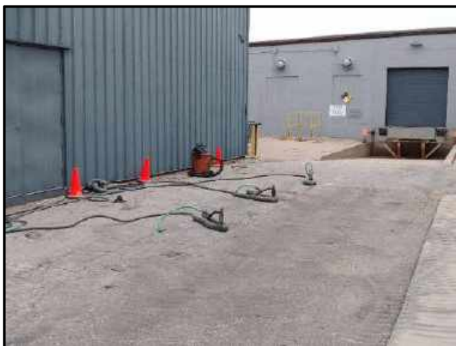
Photo 11: Active injection points in the On-Site Source Grid.
