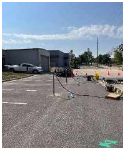
Figure 1: Active injection points in the On-site Barrier
