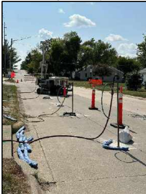
Photo 15: Active injection points in WPRB. In the background, traffic control barricades and the hydrant set up can be seen
