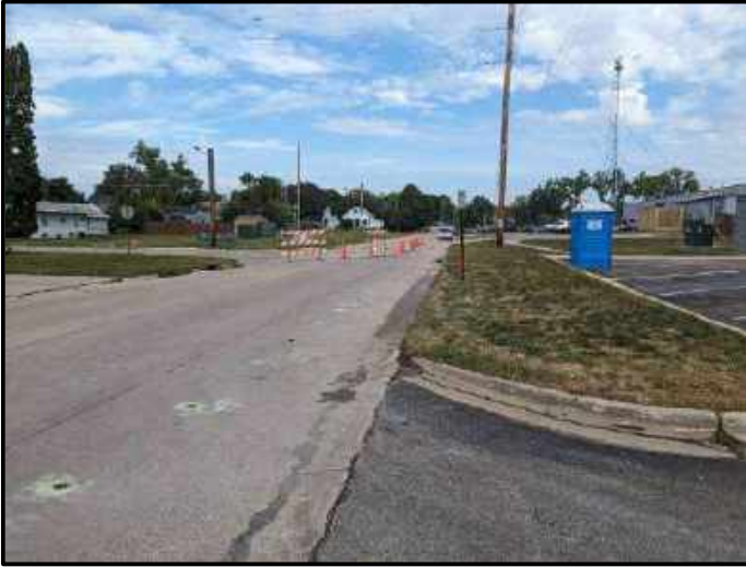
Photo 13: North section of WPRB with traffic control diverting traffic away from Eastern Ave
