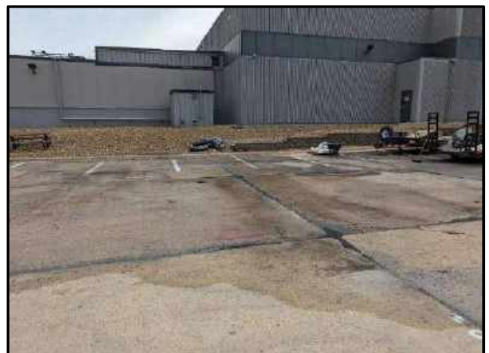
Photo 12: Injection area of the PFAS Pilot RRS had pressure washed the surface
