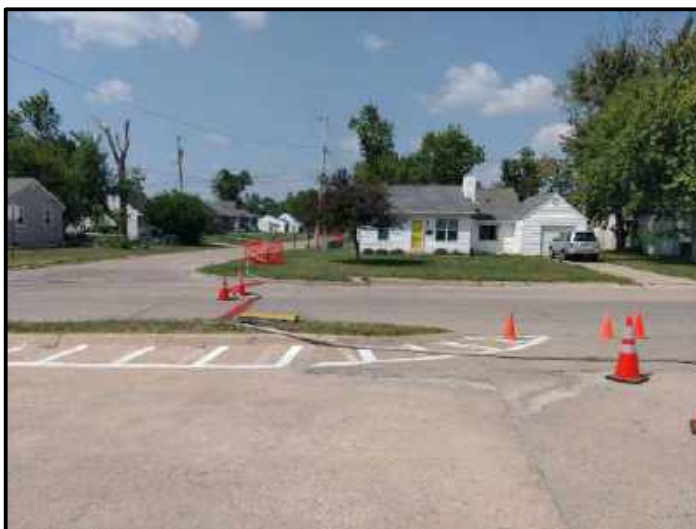
Photo 7: Firehose crossing Eastern Ave, utilizing hose ramps to supply RRS injection trailer with mixing water.
