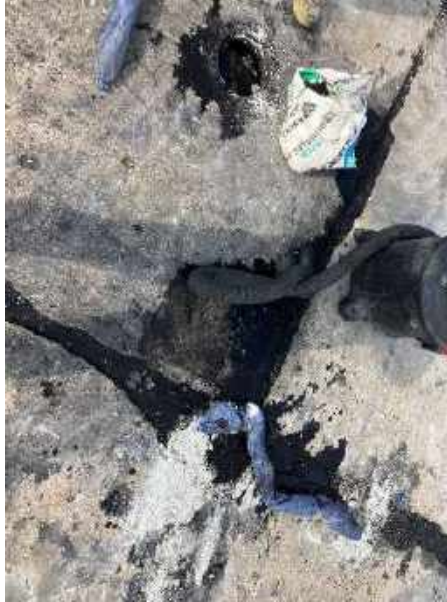
Figure 4: Daylighting episode surfacing through cracks in concrete.
