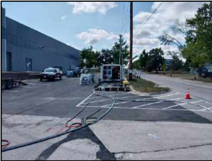
Photo 9: RRS trailer 16 set up in the southern section of the parking lot running injection lines to the PFAS Pilot
