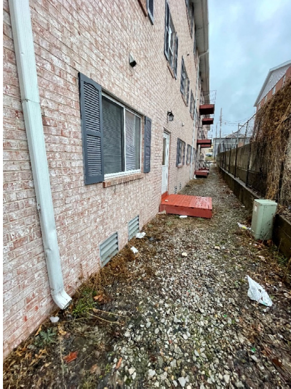
Photo 3: Passive ventilation system components at the building that was maintained with minor debris nearby.
