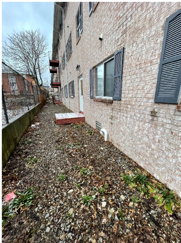
Photo 4: Typical vent and louver seen at the south partition of crawl space.
