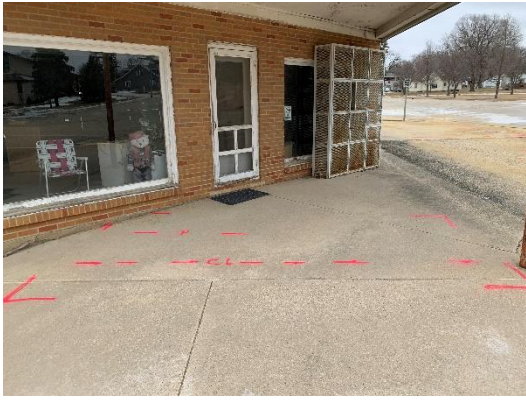
Area 1: showing center line of disturbed ground (CL) and potential piping in place (P).
