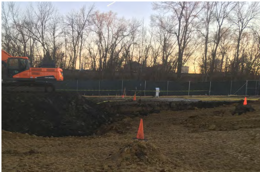
Photo 2 – Shallow excavation and backfill near where former building was located (MW-1 in foreground, MW-2 behind MW-1, and MW-3 on right, all marked with traffic cones; facing SSE).
