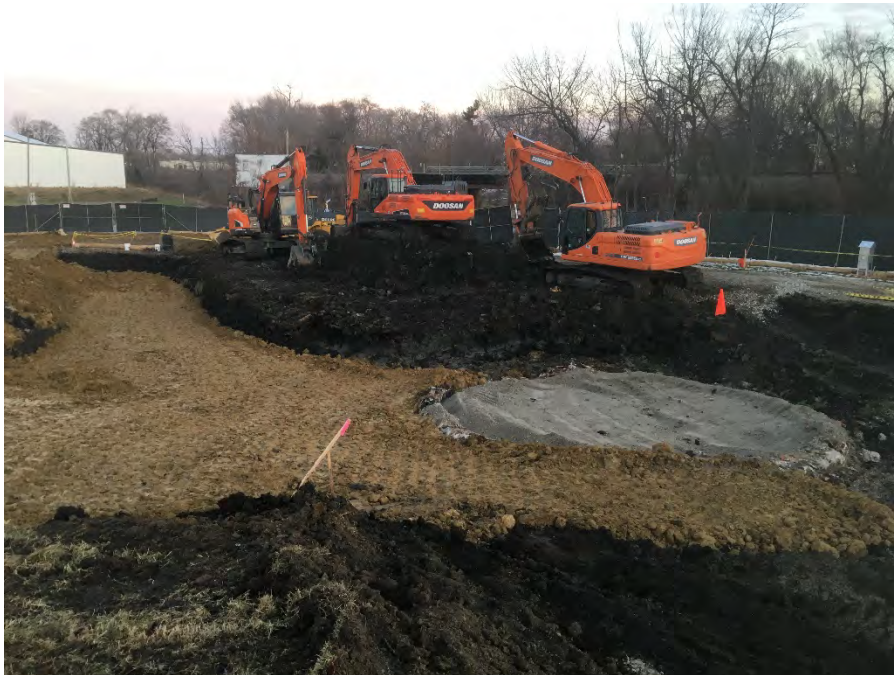
Photo 4 – Backfill along north and west sides of former building; relief holder walls removed to three feet bgs and backfilled to 3' bgs with limestone gravel. Black dirt on left side of photo is un-excavated soils near monitoring well MW-1 (facing east).
