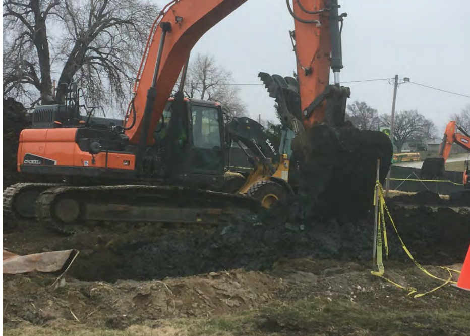
Photo 3 – Relief holder contents temporarily excavated for benefit of IDNR viewing. Material immediately placed back into holder and covered with less impacted waste soils to minimize volatilization/air impact (facing NE).
