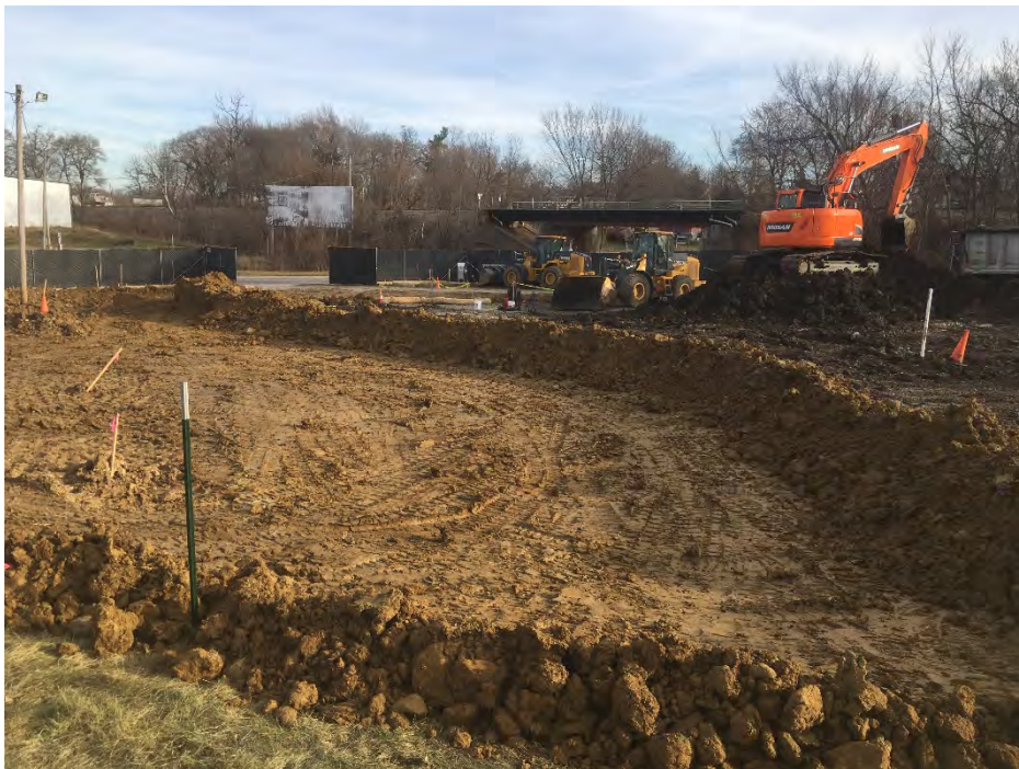
Photo 4 – In preparation for forecast rain on Friday, berms of clean fill were placed at perimeter of excavation to prevent overland flow into excavation from north and west, and to prevent impacted sediment/water from entering from south (facing SE). Berms also placed to prevent flow into relief holder (not shown in this picture)
