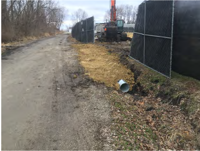
Photo 5 – Replaced culvert beneath south drive (will eventually be covered with gravel; facing WSW).
