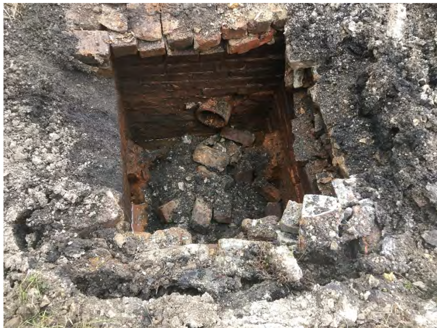
Photo 2 – Inside manway located on south edge of property to the southeast of former building. Tile shown in photo goes toward building (facing NW).
