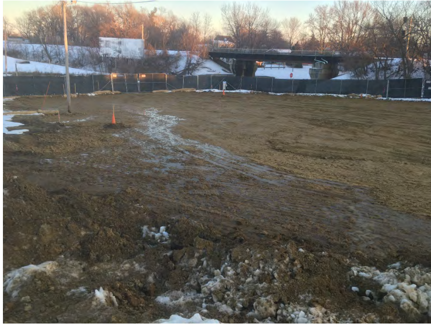
Photo 3 – Meltwater from snow piles shown in photo 2; flow is toward east side of site near original driveway (facing SE).
