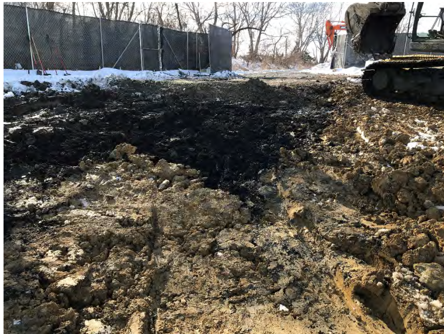
Photo 2 – View of excavation near southern extent of excavation (near D8); clean fill in foreground (facing SW).
