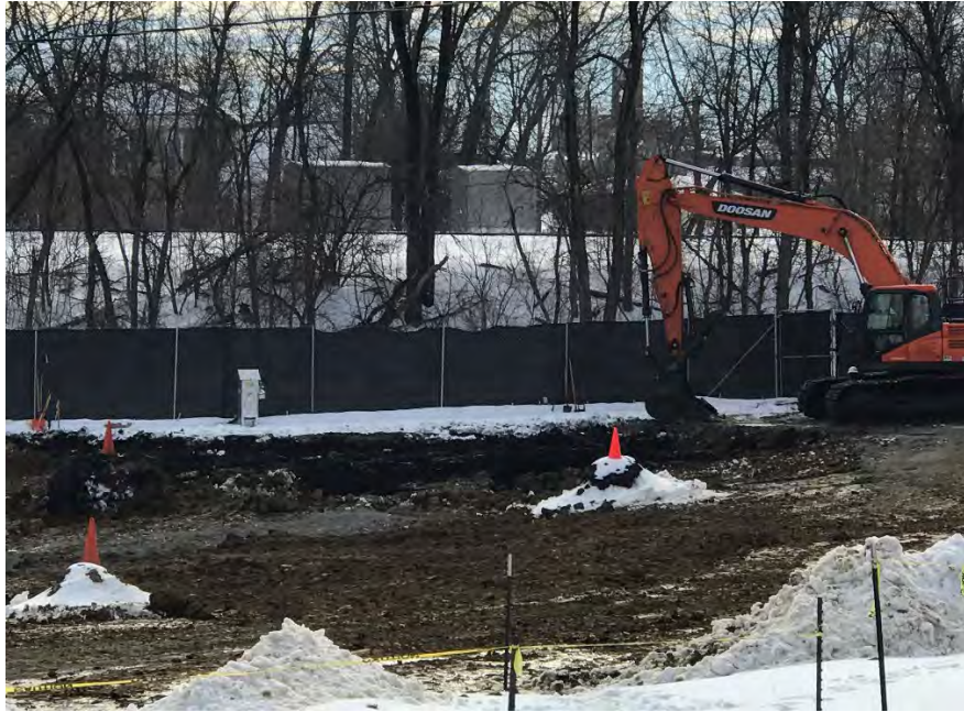
Photo 3 – View of excavation near southern extent of excavation; clean fill in foreground as well as monitoring wells MW-1(left cone), MW-2 (behind MW-1), and MW-3 (right cone; facing south).
