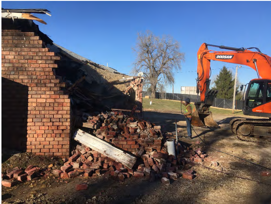
Photo 2 – Demolition of former gas plant building. Water spray used to help control dust (facing North).
