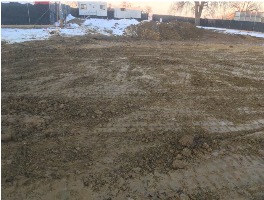
Photo 2 – View of backfilled excavation near northern area of excavation. Piles are snow cleared from excavation following holiday break with backfill melt-out (facing north).
