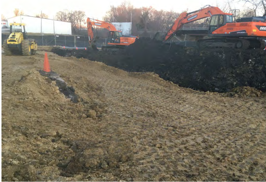
Photo 3 – Shallow excavation and backfill south and east of MW-1 (cone on left; facing E).
