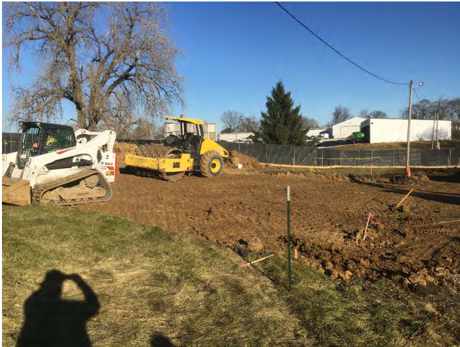
Photo 4 – Clean fill placed on northern extent of excavation. Vibratory sheep foot compactor is being used for compaction (facing east).
