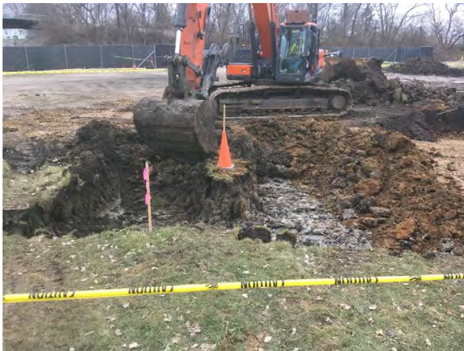
Photo 2 – Excavation in vicinity of G3. Monitoring well MW-05 under cone (facing south).
