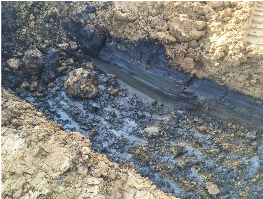
Photo 3 – Relatively un-impacted native clay immediately below (5' depth) wooden box culvert. Appeared that clay fractures had trace DNAPL presence (facing SW).
