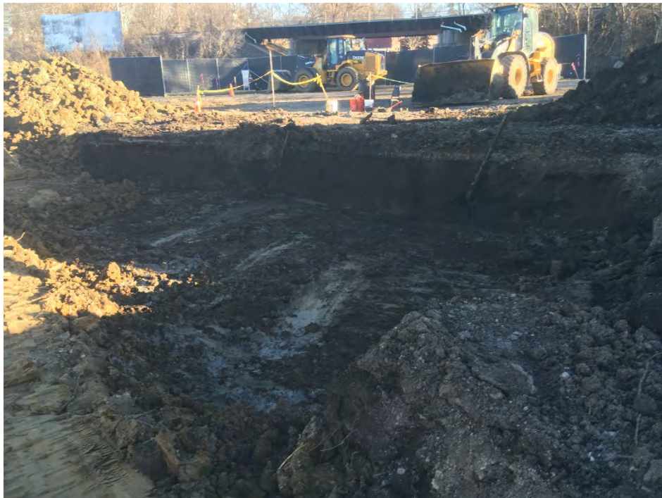
Photo 5 – Excavation near E4; lighter soil colors at bottom of excavation are very tight clays (facing SE).
