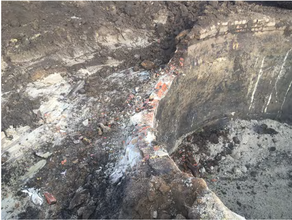
Photo 5 – West side of relief holder as upper 3 feet of holder wall is being removed. Wall remains very structurally sound. Limestone fines visible in bottom of holder (wastes dropped into holder removed prior to additional backfill placement; facing NNW).
