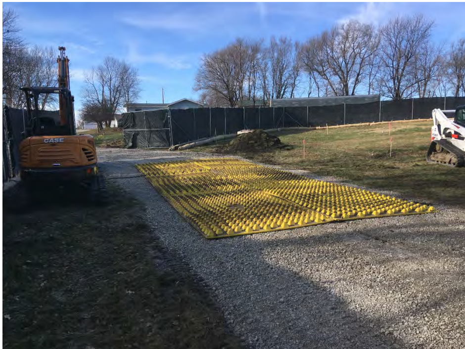
Photo 2 – Tire-cleaning mats installed in truck decontamination area along south side of site (facing W).
