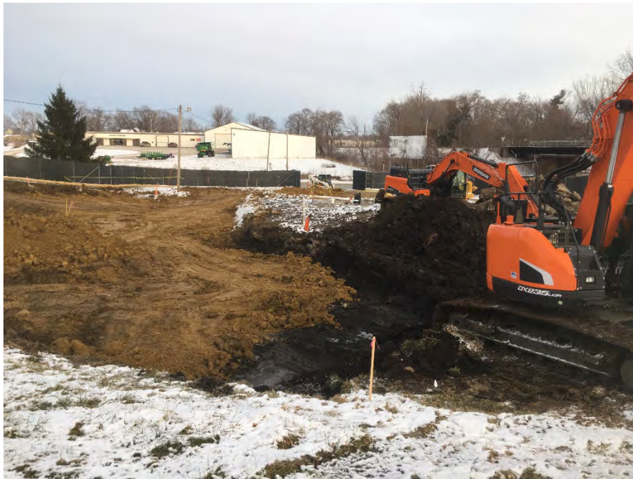
Photo 3 – Backfill on northern portion of excavation and shallow excavation NW of building (west of monitoring well MW-1 [under cone in middle of photo]; facing east).
