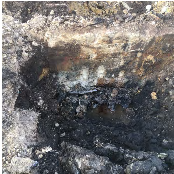
Photo 7 – Impacts/trace NAPL along outside edge of building foundation – depth at bottom at about 3.5' bgs (facing east near NW corner of former building).
