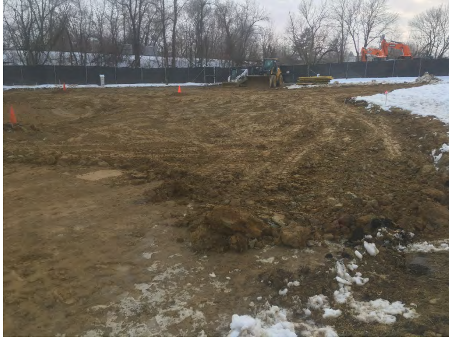
Photo 1 – View of western half of site where backfill of clean fill is at approximately 0.5 feet below original grade (monitoring wells 1, 2, and 3 under cones from left to right; facing SW).
