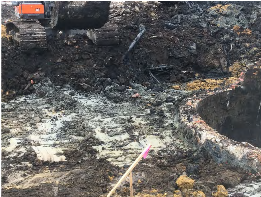
Photo 8 – Bottom of excavation where surface soils have transitioned to clay... brown hues north of the holder (foreground) transitioning to blue-green hues closer to building – depth approximately 4' bgs (facing east).
