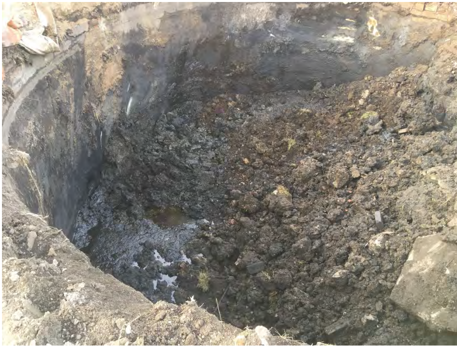
Photo 3 – View into relief holder – approximately 70% of contents have been excavated (later in the day; facing NW).
