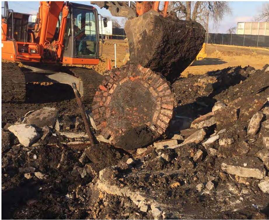
Photo 7 – Brick structure uncovered below former building floor on western half of building, east of holder. Soil beneath had minimal impacts (facing NNE).
