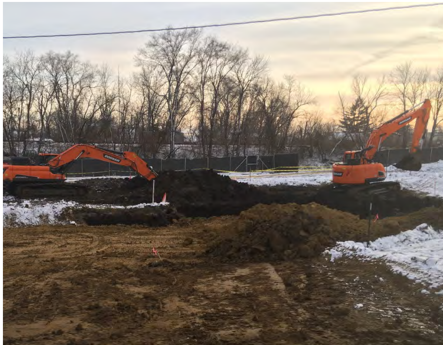
Photo 4 – Backfill on northern portion of excavation in foreground and shallow excavation NW of building (facing south).
