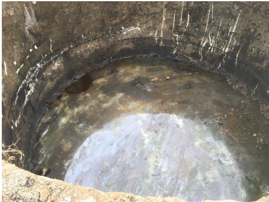
Photo 4 – After sitting empty overnight, the relief holder accumulated approximately 2 inches of water, with a couple spots where a near neutral density NAPL accumulated (left side of photo). Water was absorbed with waste soil bound for offsite disposal prior to start of backfill with limestone fines (bottom 1 foot) and ¾-inch minus limestone gravel (for compaction characteristics; facing north).
