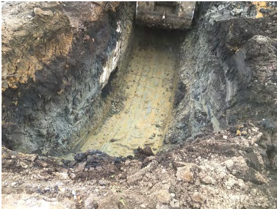
Photo 3 – Exploratory trench on east side of holder to 12 feet bgs. Concrete protrusion on holder (left side of trench) did not have any piping leaving it, and soil appeared to be native below approximately 4 to 6 feet bgs (facing north).
