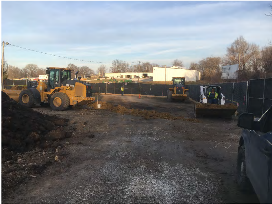
Photo 5 – In preparation for forecast rain on Friday, storm water wattles placed across gate at end of day. Berms of fill placed downslope of excavated materials to prevent runoff of impacted sediment/water.
