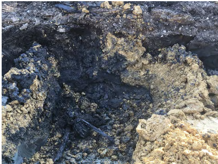
Photo 4 – Wooden box culvert within excavation cut (yet to be excavated; facing SSE).
