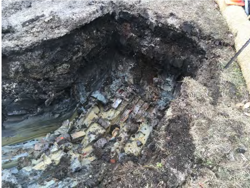
Photo 3 – Excavation of manway shown in photo 2, showing impacted soils at depth of approximately 3 feet bgs (facing SE).
