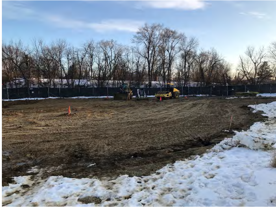
Photo 1 – View of western portion of site with clean fill to approximately 0.5 feet below grade (facing SW).
