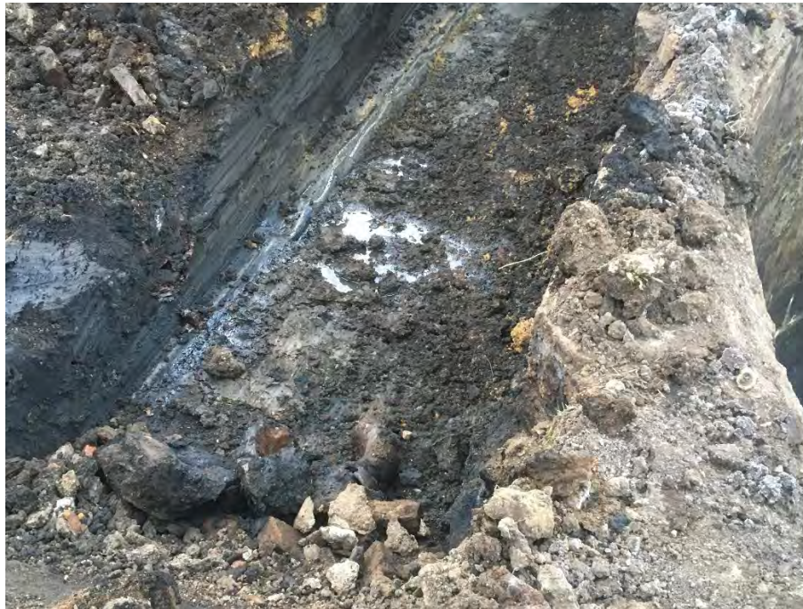
Photo 2 – Shallow (3 foot bgs) impacts along east side of relief holder. Steel pipe along left side of trench (see scrape marks from bucket teeth) fill with water and trace DNAPL (facing SSE).
