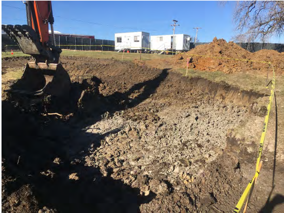
Photo 3 – Excavation near F3 on site grid; very tight clay at base of excavation (facing NW).
