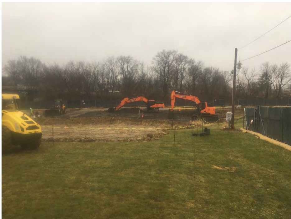
Photo 2 – View of work area at end of day on Friday (early shut down due to rain - facing south).
