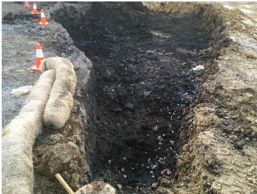
Photo 4 – Shallow excavation near I4, where multiple tiles/pipes were encountered at 3 foot bgs, soil impacts significantly less at 4 feet bgs (shown, facing WSW).
