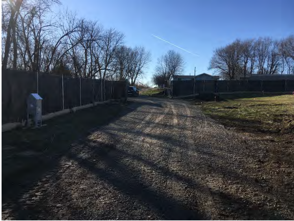
Photo 1 –View of newly constructed haul road along south side of site (facing SW).
