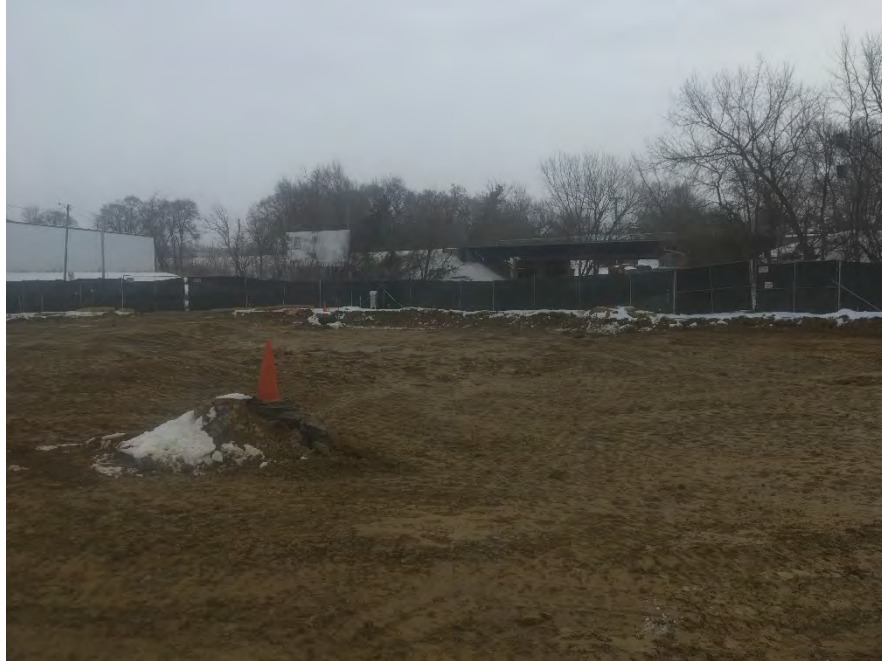
Photo 1 – View of site with clean backfill over all entire extent of excavation (facing SE).
