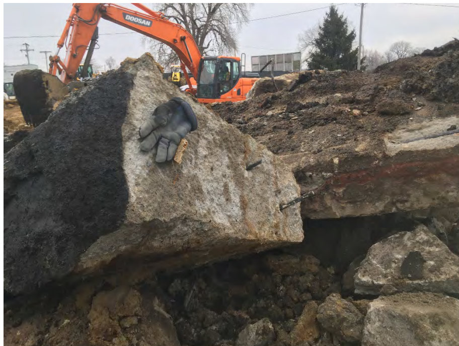
Photo 4 – Foundation materials from north side of former building; impacted black soil on bottom yet to be scraped off prior to disposal as C&D waste (glove placed on clean break for scale; facing NE).
