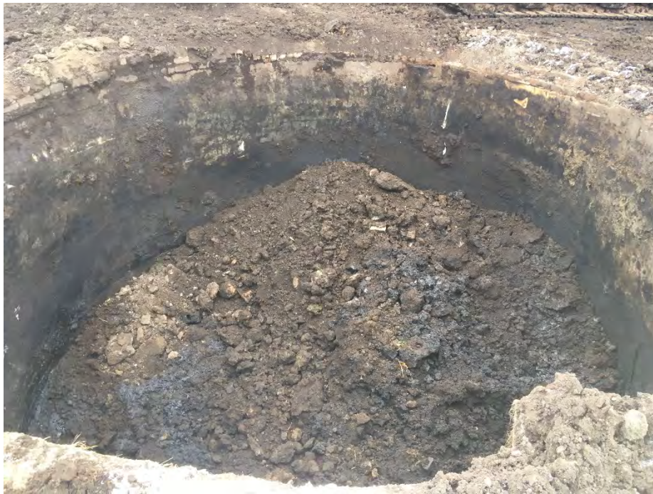
Photo 3 – Remaining contents of relief holder mid-day Tuesday. Lighter colored soils are less impacted waste soils placed on heavily impacted holder waste to minimize volatilization (facing NE).
