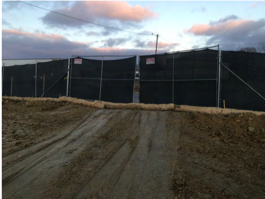
Photo 6 – Erosion wattles placed across east fence prior to extended holiday break (facing ENE).
