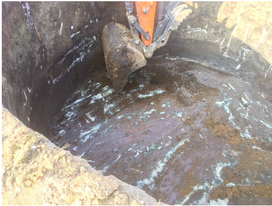
Photo 5 – Bottom of relief holder being scraped by excavator bucket with flat cutting edge. Holder was essentially watertight with negligible solids, water, or NAPL left in bottom (facing NW).
