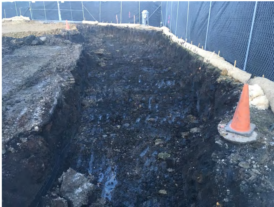
Photo 4 – Shallow excavation in southeast corner of site (MW-6 on right, facing NE).
