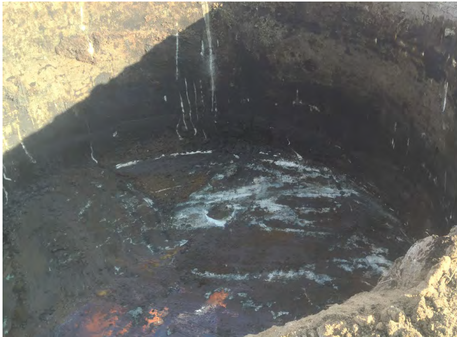
Photo 6 – Bottom of relief holder showing possible sump in eastern side of floor (dark area in middle of lighter colored scrape marks). Metal protrusion was also found in center of holder, as well as potential sump on holder floor directly adjacent to east wall (facing NE).
