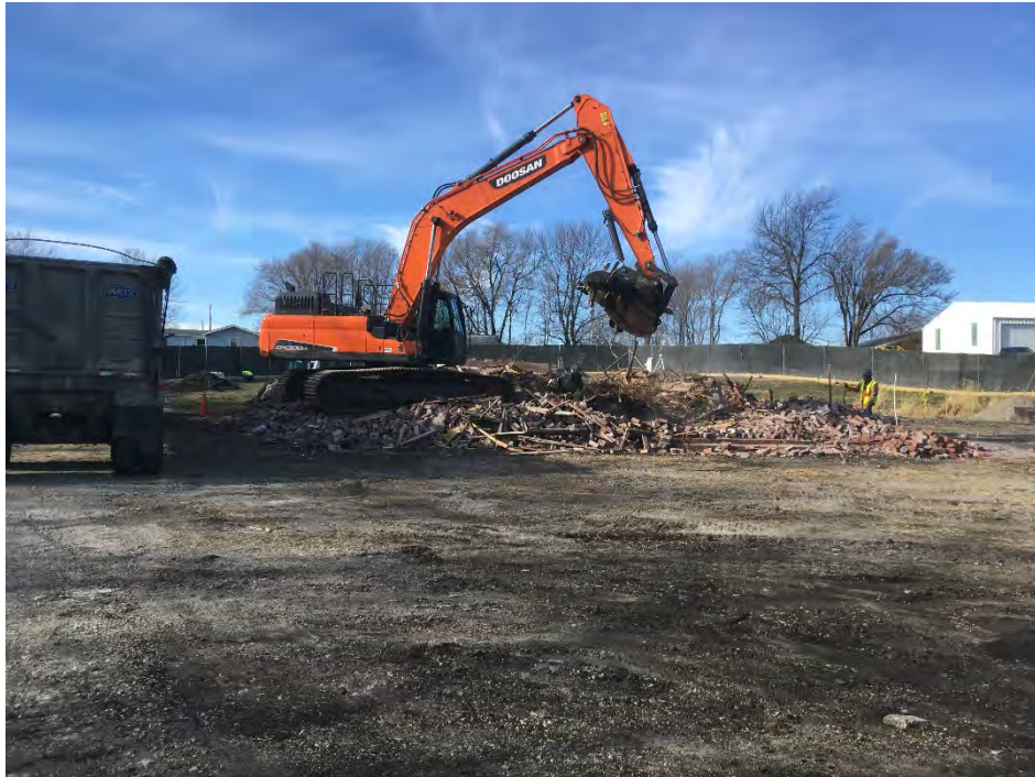
Photo 1 – Load-out of demolition debris. Water spray used to help control dust (facing NW).
