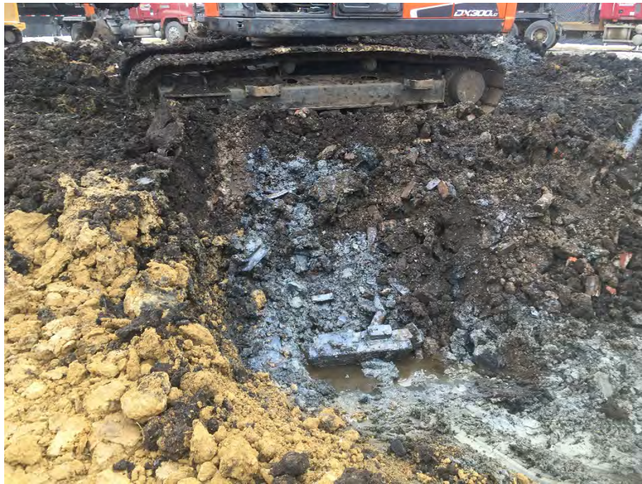
Photo 9 – Brick structure at depth of approximately 5' bgs near NW corner of building, associated with clay tile that extends north to south in this area. Clay tile was full of water/trace NAPL leaving strong sheen on soils in this area (facing SE).
