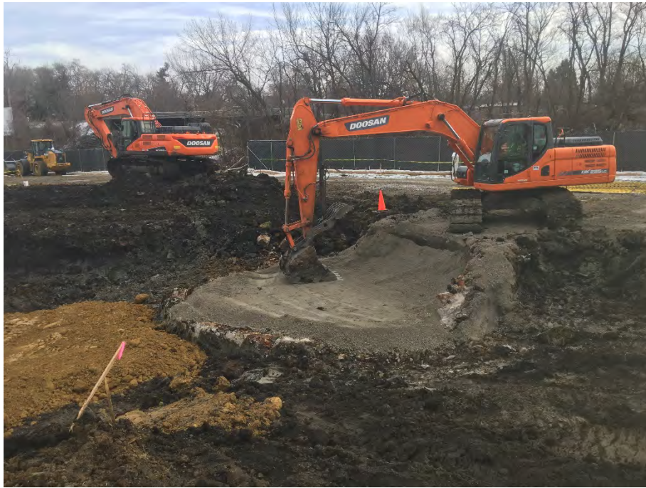
Photo 3 – Backfill and compaction with bucket of relief holder. Walls on west, north, and east sides have been removed to approximately 3 feet bgs. Holder was backfilled with an initial 1-2 foot layer of limestone fines (3/8" minus), followed by 3/4" minus limestone gravel to 3 feet bgs. Clay backfill will be used to near original grade (facing SE).
