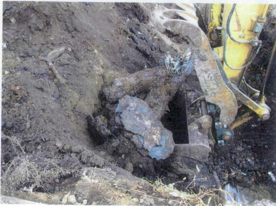
View is of the debris and logs being removed from the north side of the tanks. Broken glass, bottles, bricks, and plastic pieces can be seen at the bottom of the trench to the right in this photo.
