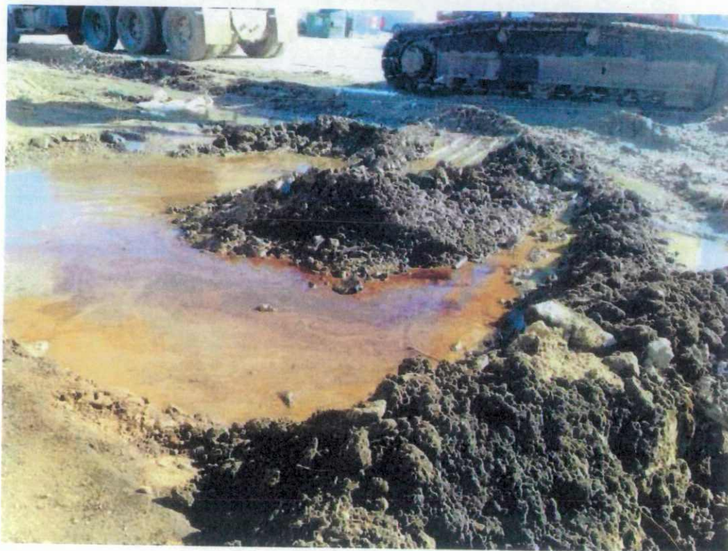
View is of the south side of the tank system. The berm soil was pushed into this area to absorb the fuel and water prior to removal.
