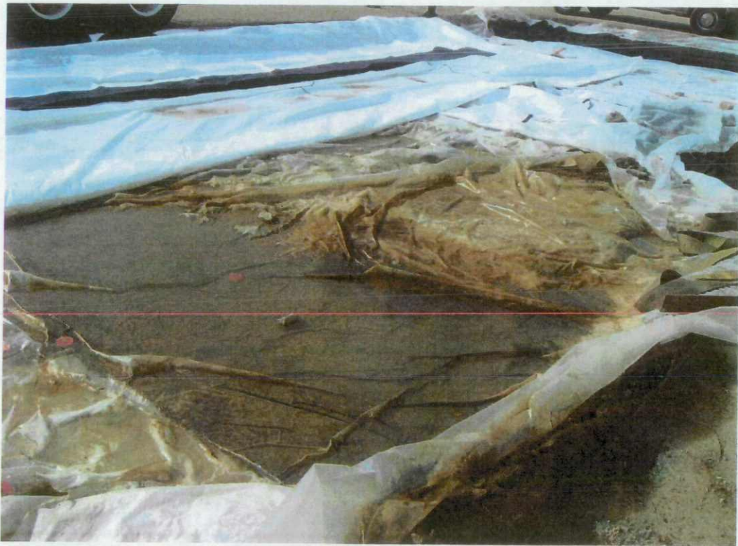
View is of the soil under the plastic on the south side of the tanks. The concrete pad is visible in the right portion of this photo.
