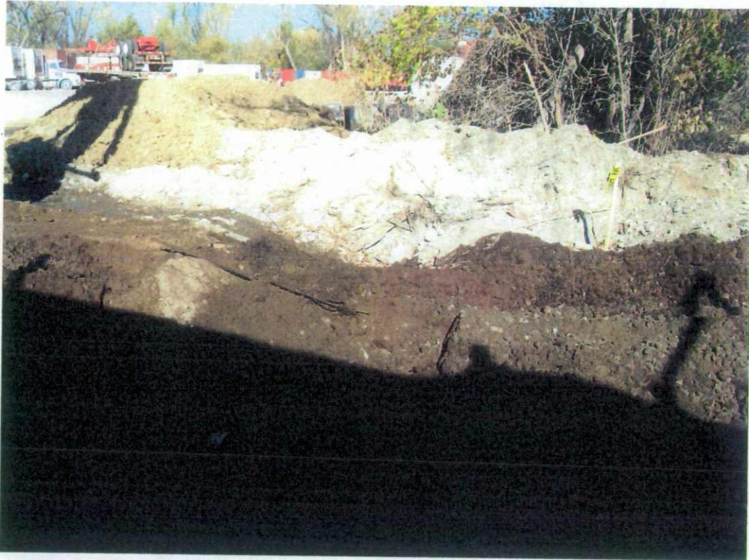
View is to the north as excavation continues. The marker showing the extent of the spill is seen in this photo. Piles of clean fill material can be seen in the upper left in this picture.
