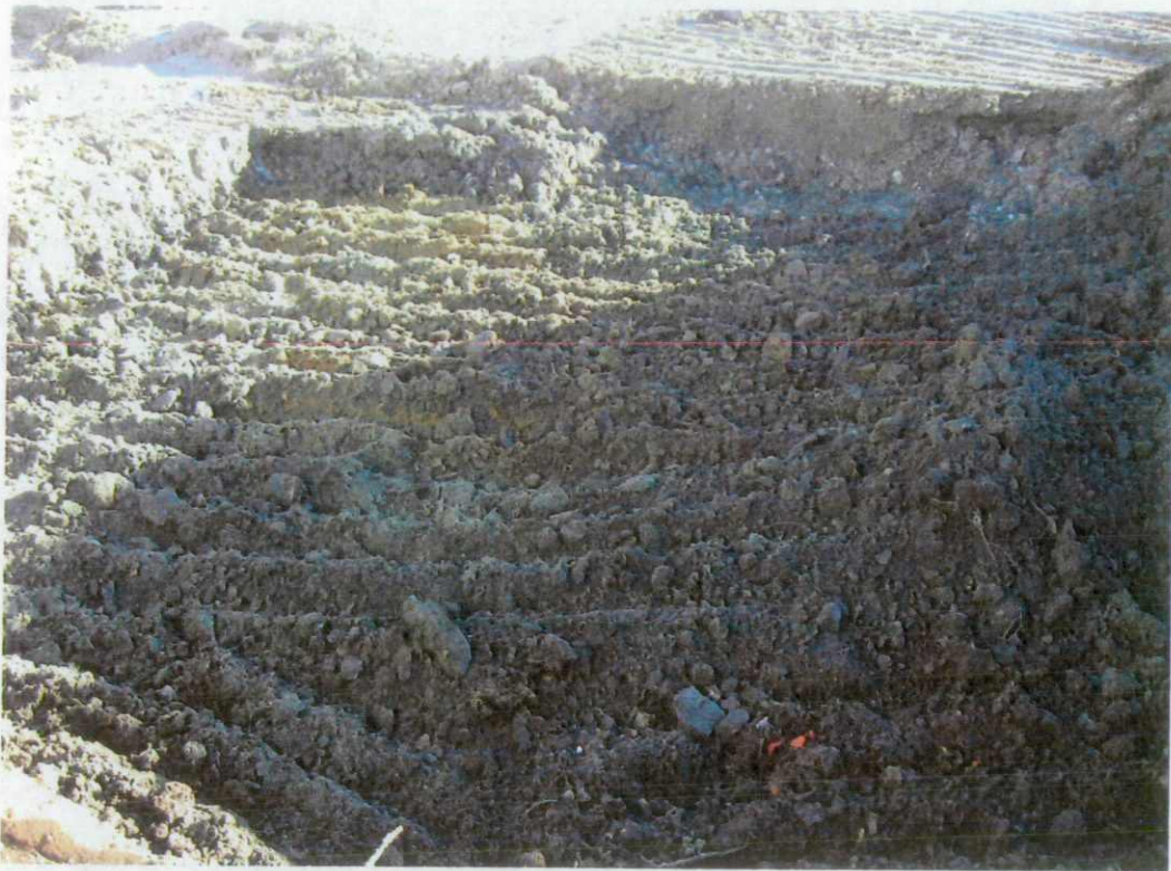
View is of the beginning of the excavation activities, as soil is removed in 2-foot increments.
