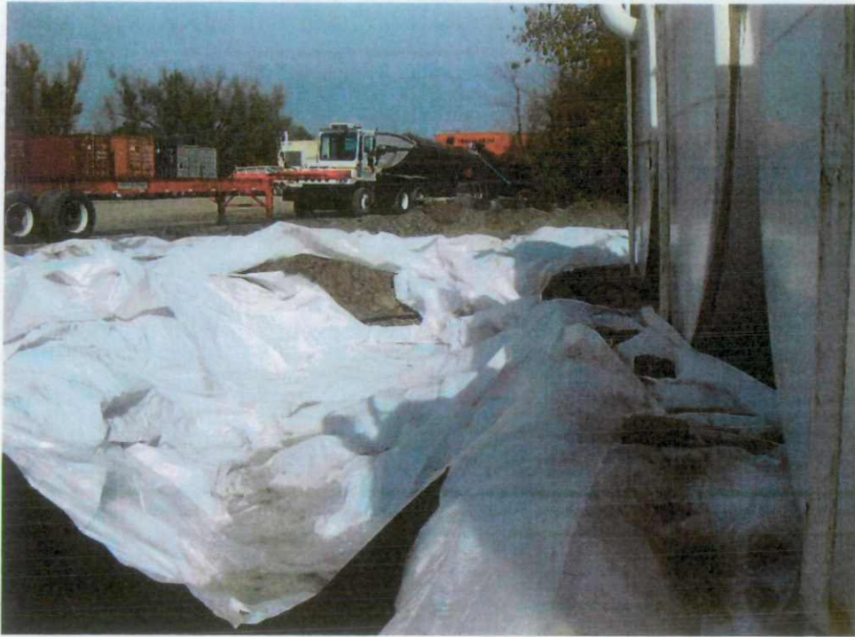
View is of the west side of the ASTs. Soil beneath the plastic was removed to approximately 3-feet at the edge of the concrete pad. The trucks holding the excavated soil can be seen in the background. The soil was eventually transported to the Pheasant Point Landfill in Douglas County.
