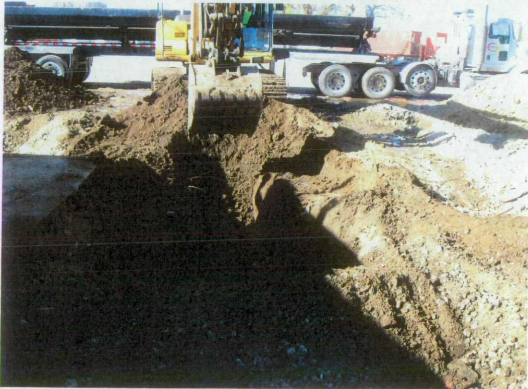
View is looking to the west as excavation continues on the north side of the tank system.
