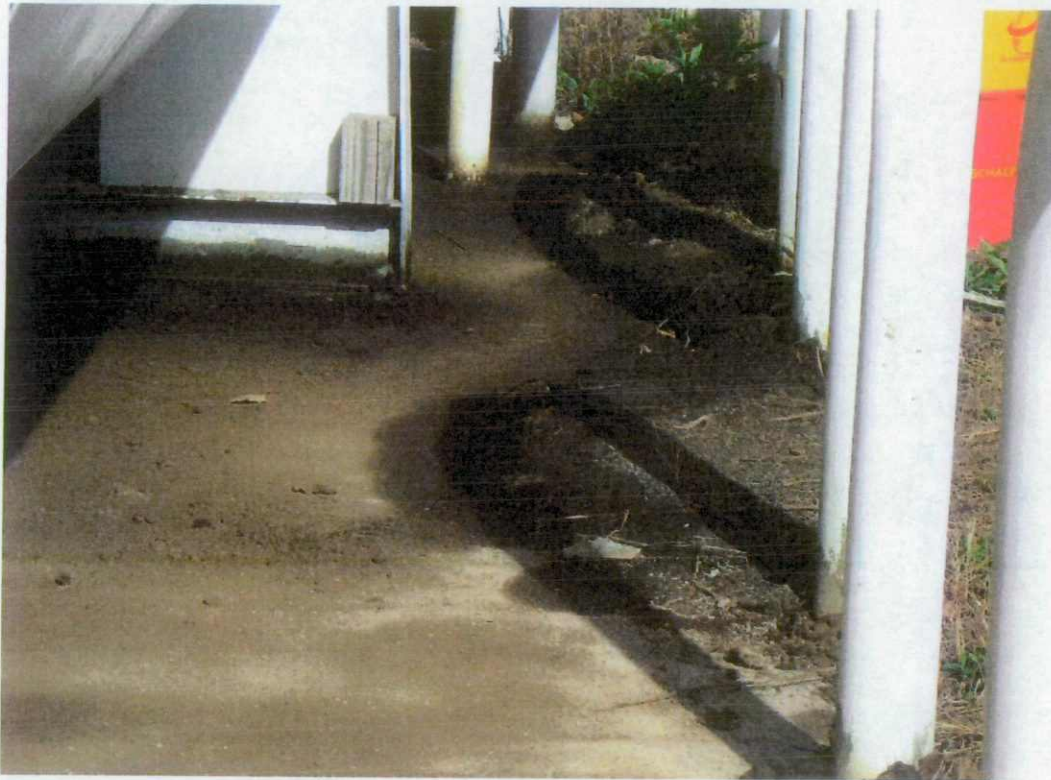
View is of the concrete pad and soil on the east side beneath the fueling station.
